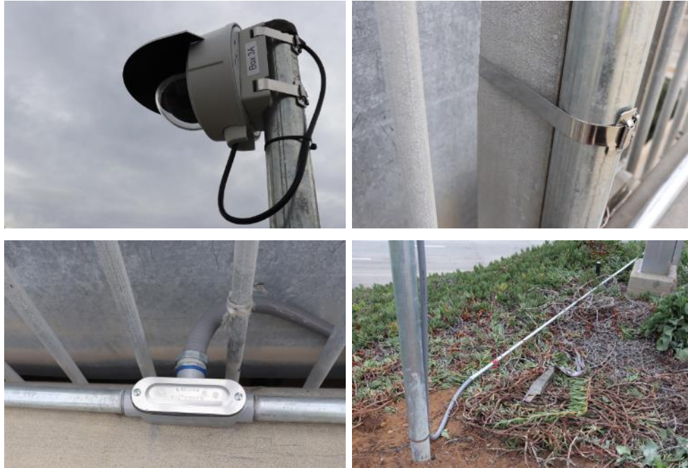
Figure A1.7: Details of camera mounting and cabling at Las Flores Overcrossing
