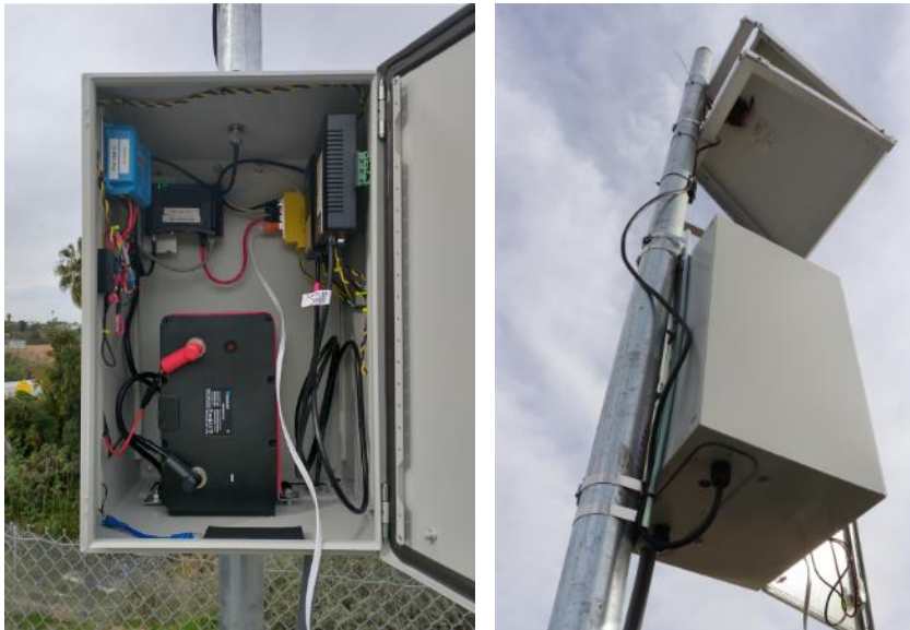
Figure A1.5: Pictures of electronics box and solar panel
