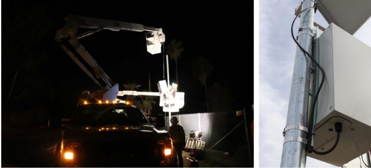
Figure A1.8: Left: Installation of electronics box at Jefferson Overcrossing with a bucket truck; right: straps around the steel pole.
