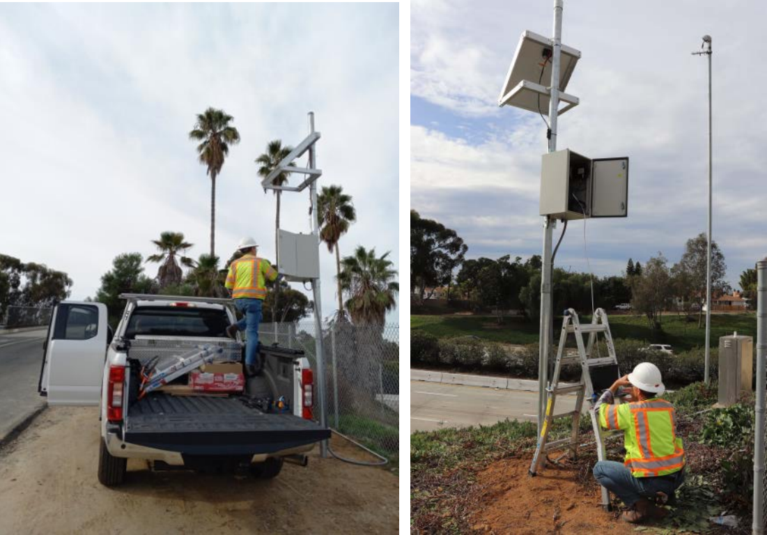
Figure A1.9: Access to electronics box: Left: at Jefferson Overcrossing, Right: at Las Flores Overcrossing.
