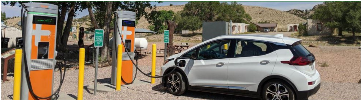
► (Above) A DC fast charger in use at the Dinosaur Welcome Center in Dinosaur, Colorado. Photo credit: Colorado Department of Transportation
