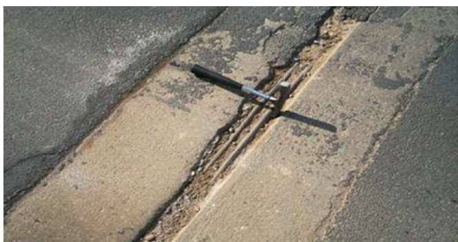
A bridge joint packed with incompressible debris.
