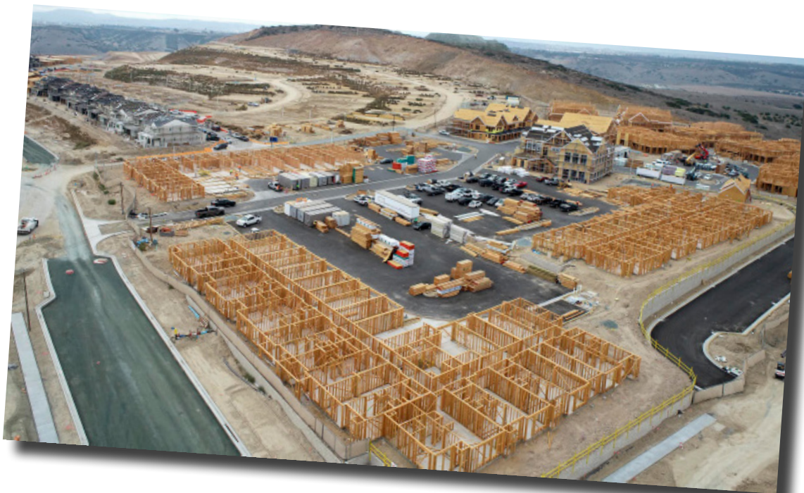
The Residences at Cota Vera are under construction. Reylenn Construction is building 280 multi-family apartment units.
