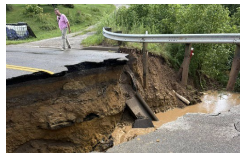
Figure 46 Example landslide washout of culvert.
