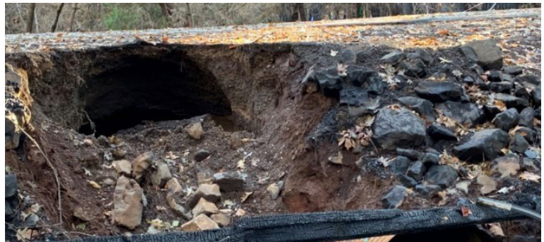
Figure 36 Collapsed melted culvert caused by the 2018 Camp Fire. (American Concrete Pipe Association, 2021).
