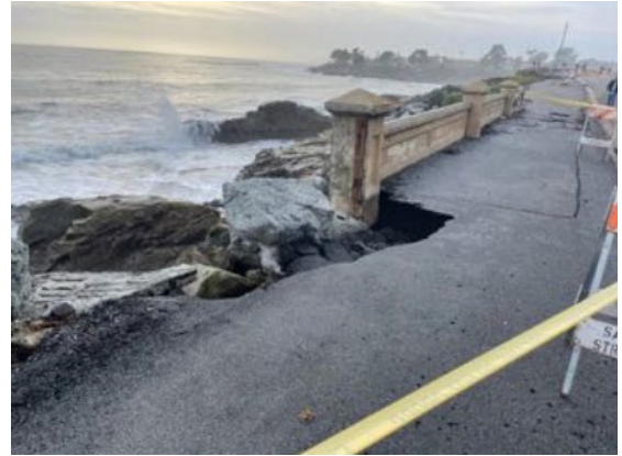
Figure 11 Bethany culvert failure in Santa Cruz County, District 5.
