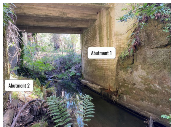
Figure 9 Bridge scour of the Boulder Creek Bridge, Santa Cruz County (District 5).
