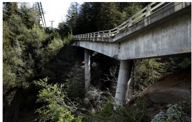
Figure 45 Landslide-related bridge failure at Pfeiffer Canyon Bridge. LA Times, 2017
