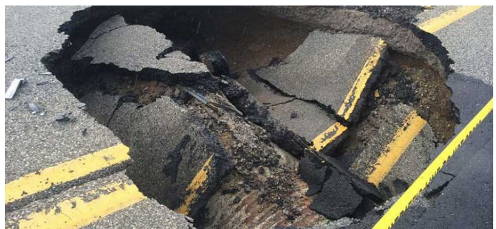
Figure 27 Culvert failure. Source: DirtWirx, 2026.
