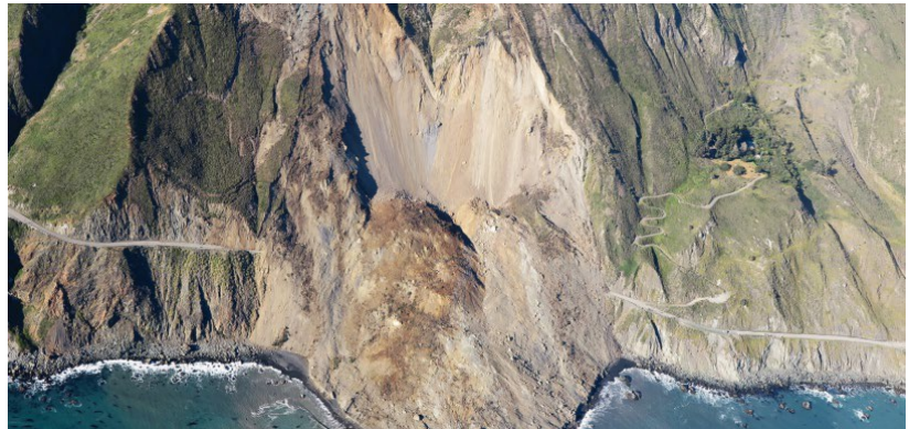
Figure 44 Example of lane failure due to slope movement in Big Sur.
