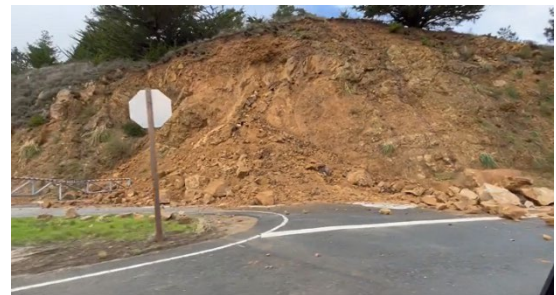
Figure 10 Slope instability near the Tom Lantos tunnels on the SF Peninsula (District 4). Source: ABC News.
