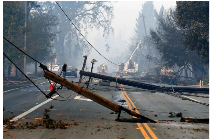
Figure 34 Downed power lines after a wildfire in Santa Rosa, District 4. Source: San Francisco Chronicle (2017).
