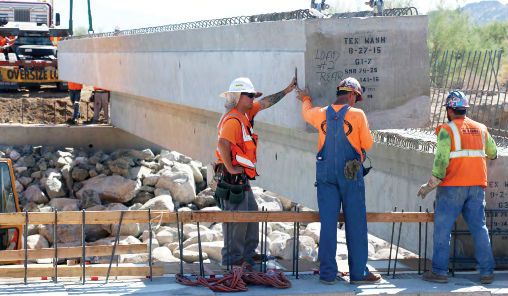
Workers guide one of 10 girders, each weighing 55 tons, during construction of the new Tex Wash Bridge.
