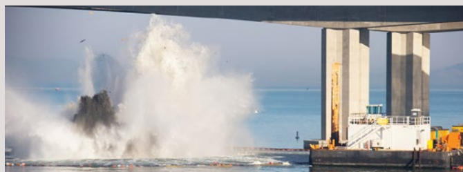
Money was saved on the implosion of the old Bay Bridge footings.
