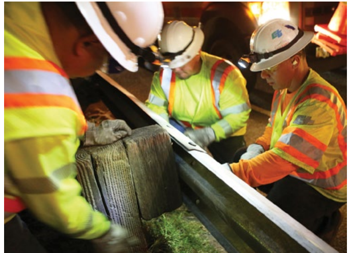
The overall condition of guardrails statewide improved significantly in 2017 from the previous year, Caltrans' Level of Service report found.
