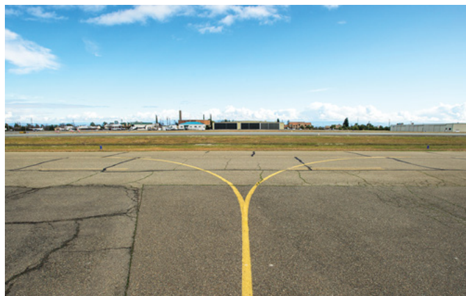
Airport pavement deteriorates over time, so inspectors with Caltrans' Division of Aeronautics perform regular checkups to ensure infrastructure at more than 400 facilities in California meets standards.
