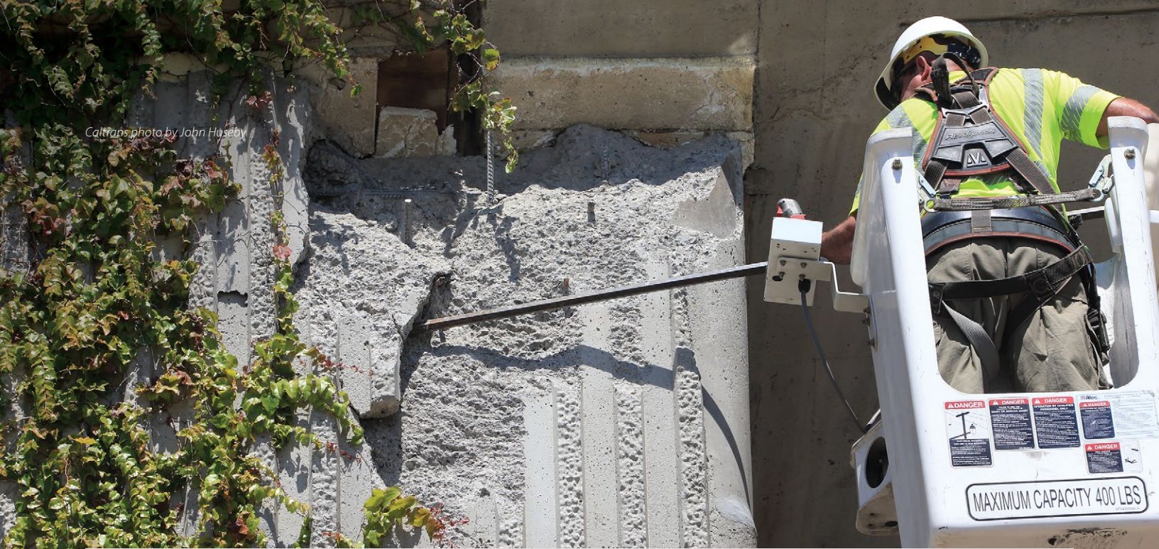
A Caltrans Maintenance employee pries off concrete from the Maxwell Bridge in Napa that was damaged by a 6.0-magnitude earthquake in August 2014. Based on the quake's intensity, Caltrans' ShakeCast system sent email alerts warning of possible damage to Department structures.
