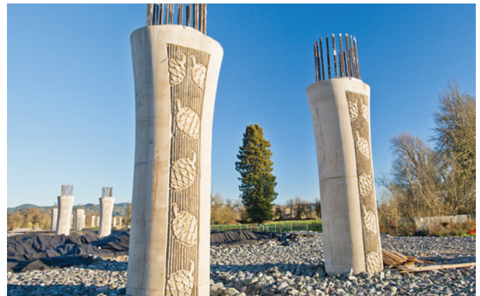
These columns, or bents, rise over 20 feet to support the 1.1 mile viaduct. In all, 64 of these columns support the viaduct's roadway.
