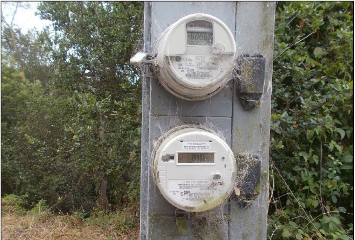
Electric meters on site
