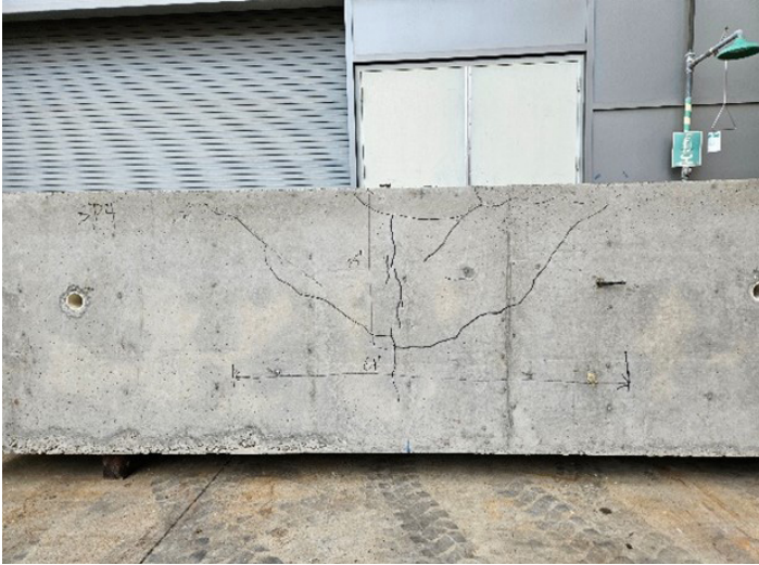
Image 2: Breakout cracks developed in a concrete beam specimen due to the tensile force exerted on the headed bar (the portion of the bar above the top face of the beam was cut off after the test)
