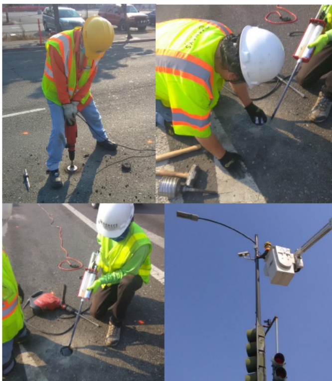
Image 1: Caltrans and Sensys installing a magnetometer and connecting it to a wireless access point
