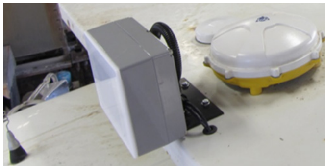
FIGURE 3: Radar, modem, and GNSS antenna installed on top of a snowplow cab protector
