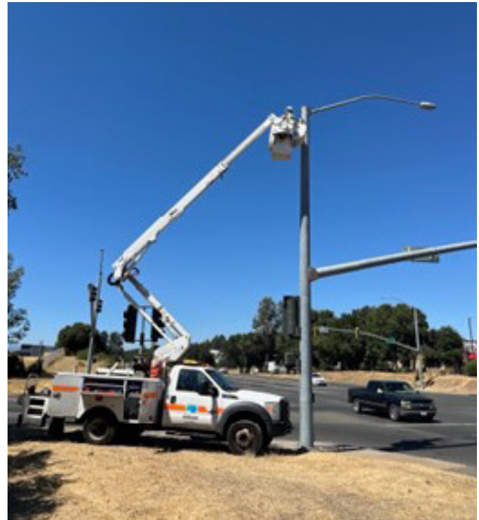
Image 2: Field staff installing camera and LiDAR equipment at Dam Rd & CA 53, Clearlake, CA.
