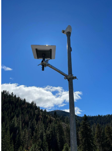
Image 2: Starlink high-performance flat antenna after installation – Image Source – AHMCT
