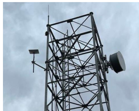
Image 1: Starlink high-performance antenna (left side of image) after installation at the Redding Fiber Hub – Image Source - AHMCT
