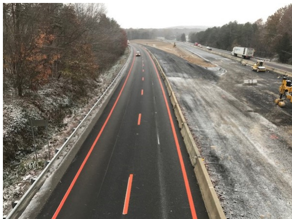
Image 4: Kentucky DOT orange temporary work zone pavement delineation
