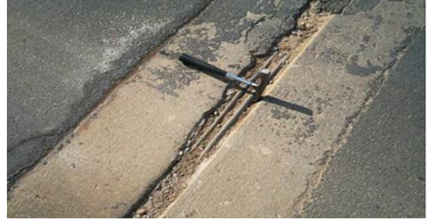
Image 1: A bridge joint packed with incompressible debris.
