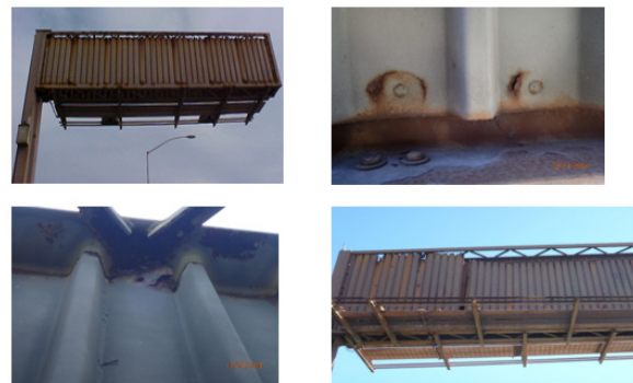
Image 1: Typical corrosion damage of in-service box beam sign structures
