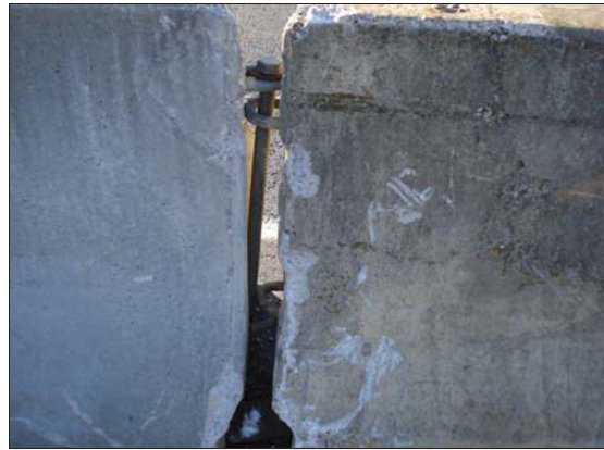
✗ Not Bolted at Bottom
