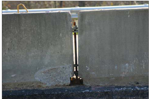
✗ Bolt Too Small (Minimum Diameter 1 1/4" Required)
