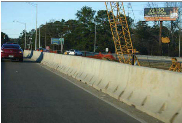
✗ No Reflectors On Top of Rail
