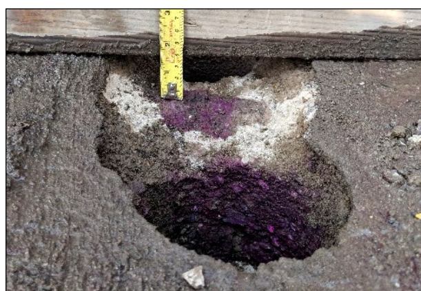
Figure 6.24: Carbonation extent beneath microsurfacing.
