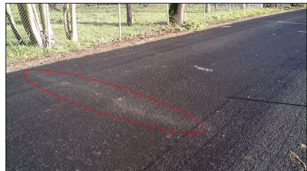
Figure 6.5: Crack identification by discoloration after water spraying.
