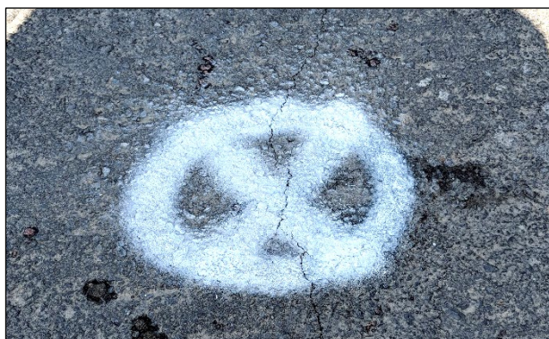
Figure 6.20: Core location through shrinkage crack.
