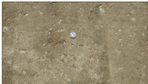
Figure 5.32: Close-up of microcracked surface.
