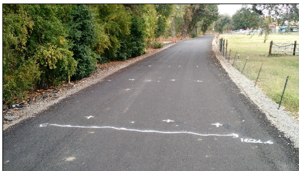
Figure 6.6: Marked crack with location.
