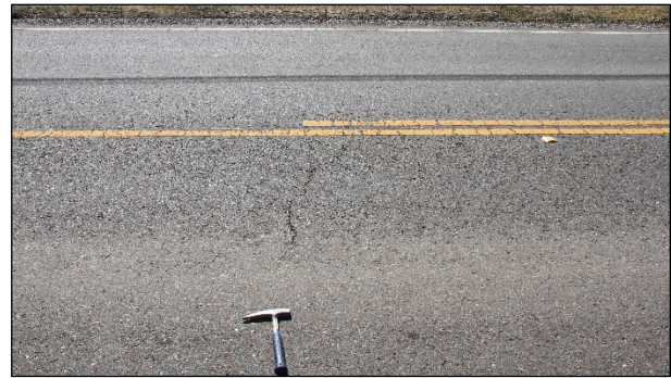
Figure 2.2: CR32B: Example transverse cracks.
