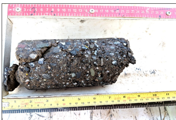
Figure 6.22: Core taken across shrinkage crack.
