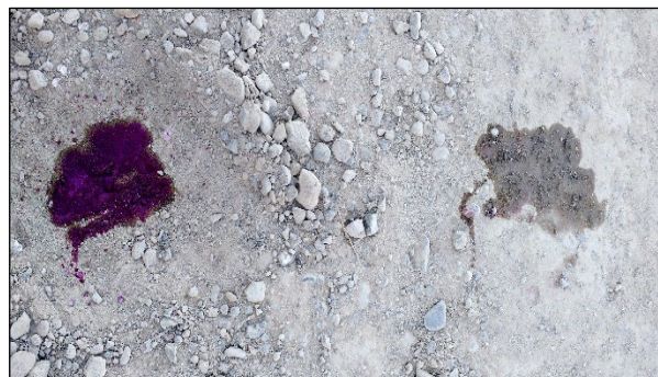
Figure 3.5: Surface carbonation on an FDR-C layer.
