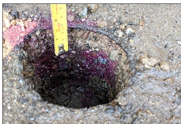
Figure 6.23: Carbonation with depth in core hole.
