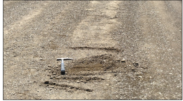
Figure 2.15: Sliver fill damaged by microcracking.
