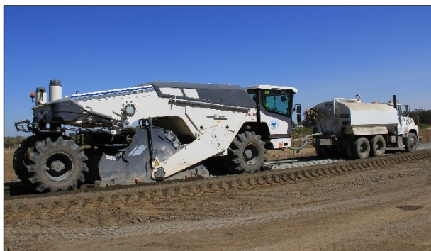
Figure 5.6: Water tanker and reclaimer.
