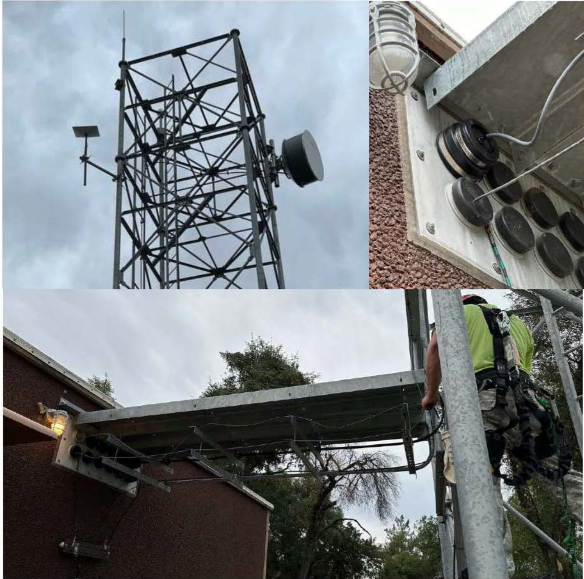
Figure B.3: HP Starlink mounted on the Hub tower (Courtesy of District 2)
