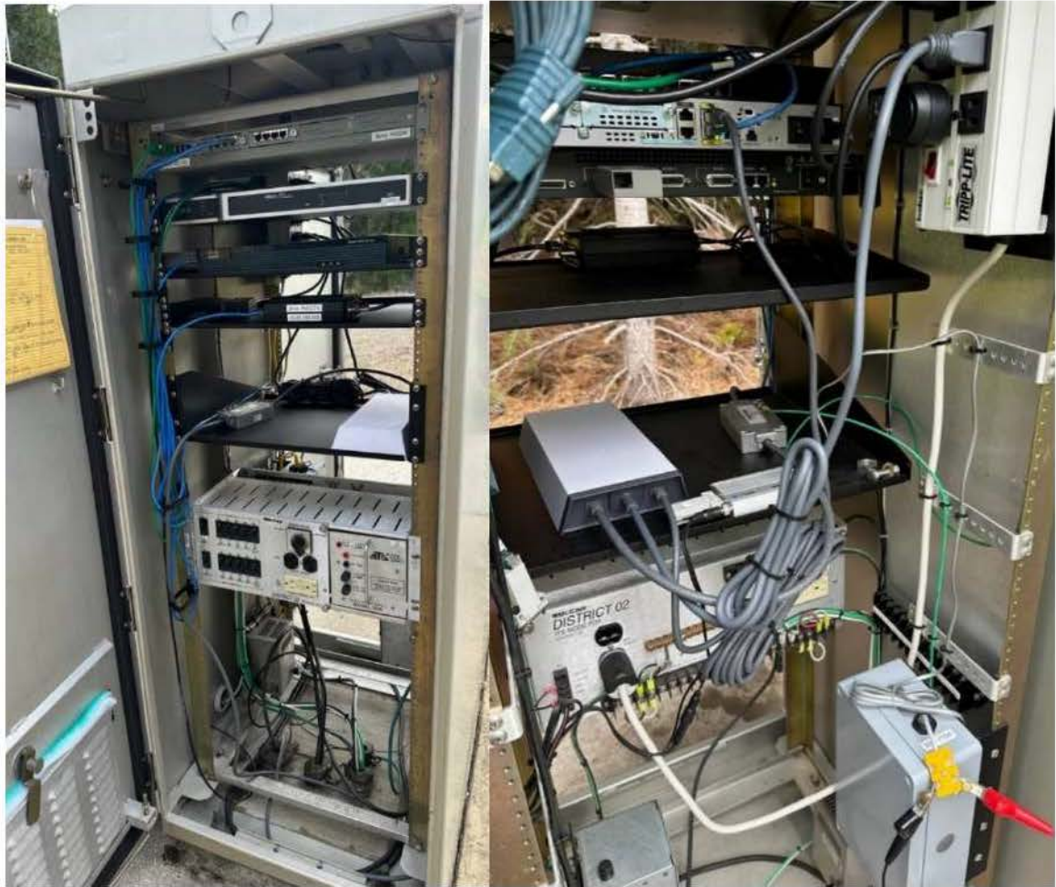
Figure B.5: Starlink power supply and PolyPhaser surge protector housed temporarily in highway cabinets next to CCTV poles (Courtesy of District 2)
