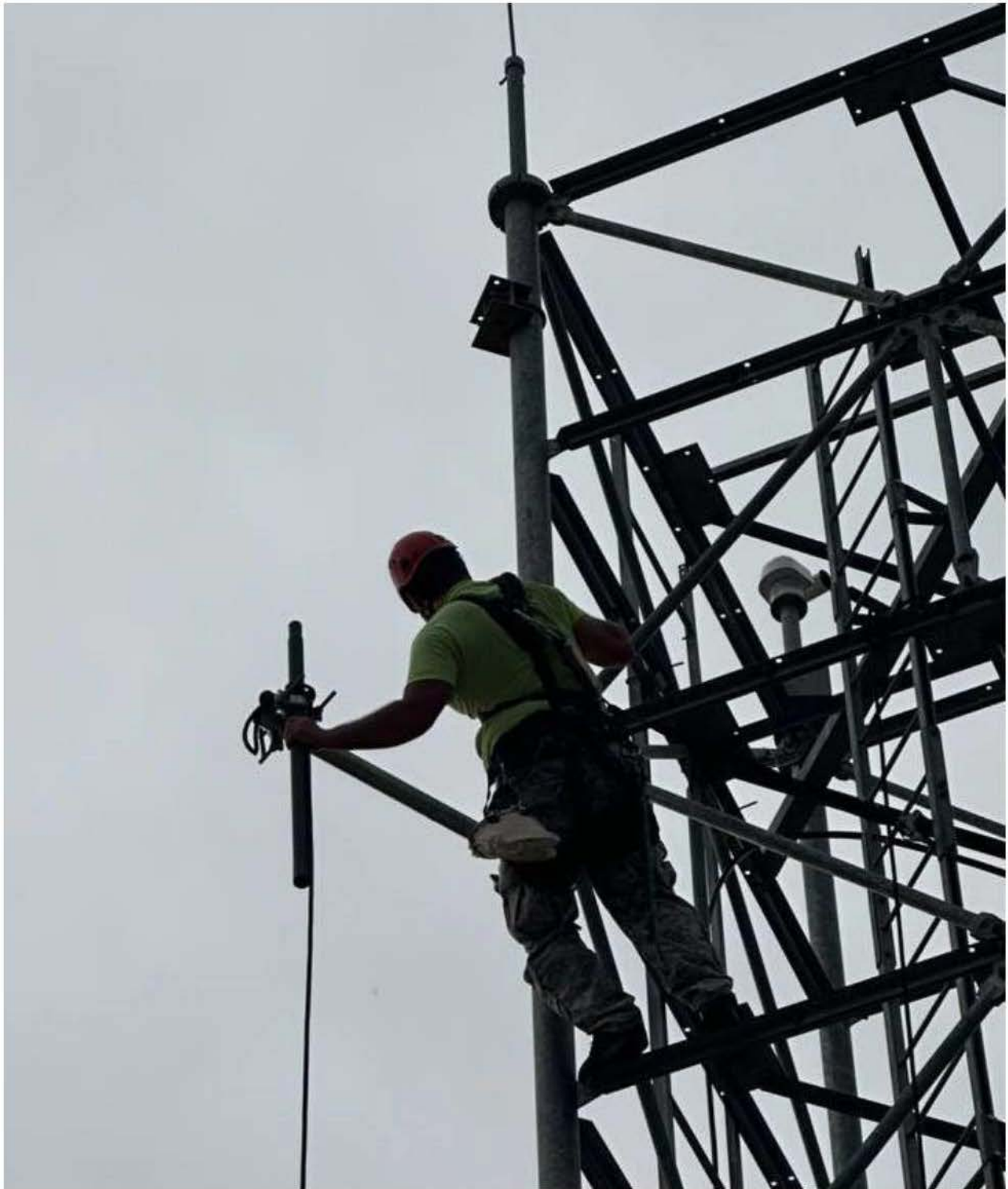
Figure A.13: The top half of Starlink Ground Pole being installed at Redding Fiber Hub as the base for the actuated HP antenna
