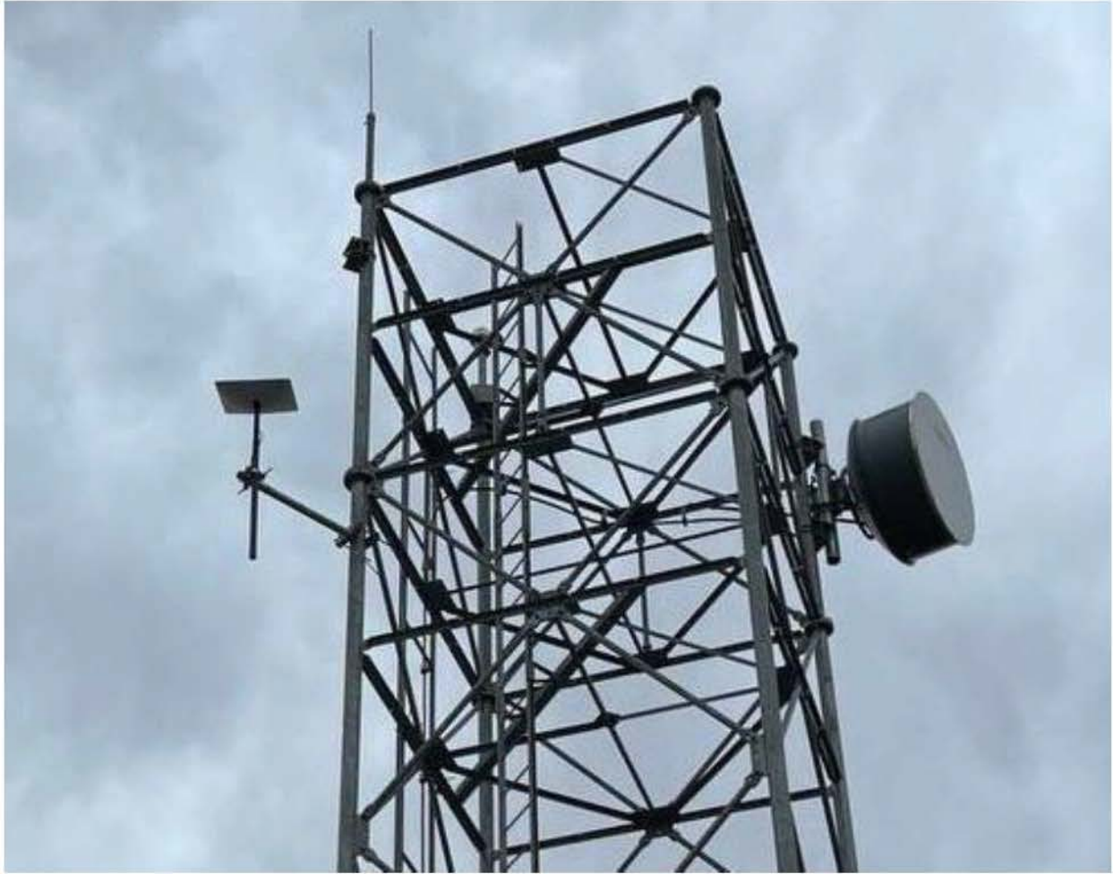
Figure A.14: Starlink Ground Pole after installation at the Redding Fiber Hub
