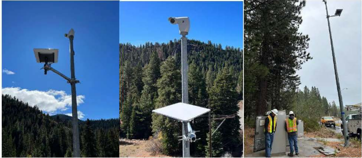
Figure B.4: Flat HP Starlink mounted on CCTV pole (Courtesy of District 2)
