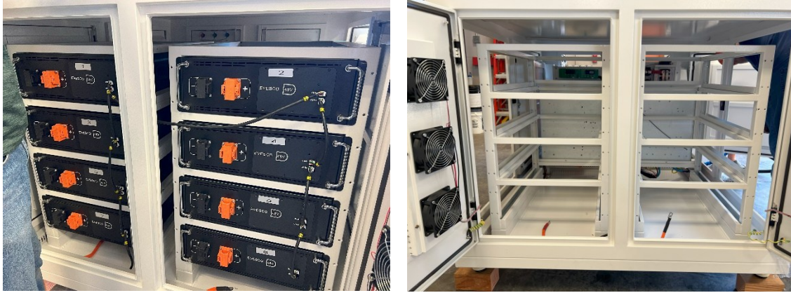
Figure 3.4: EVES-6060-NA interior and battery modules mounted
