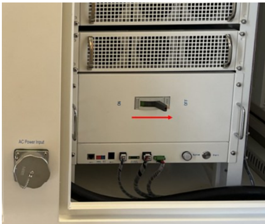
Figure B.6: Turning the master control switch to "OFF" before closing and locking the unit
