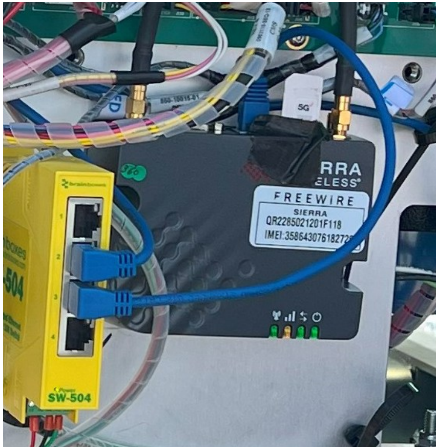
Figure 3.18: Sierra Wireless MP70 installed on Caltrans' FreeWire Boost Charger 200. After setup, the modem showed a solid green network and Wi-Fi LEDs. The activity LED was flashing amber, indicating that data was being transferred successfully via the ethernet port.
