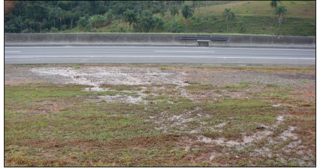
Figure 3.33: Water flowing downslope into the road.
