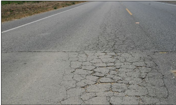
Figure 3.22: Early failure in patch (drainage problem).
