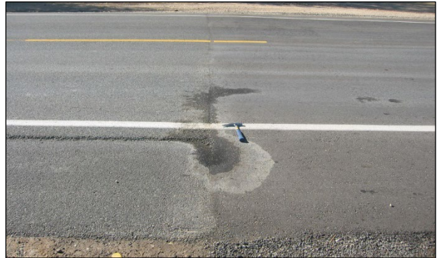
Figure 3.23: Early failure in patch (note water pumping in joint).
