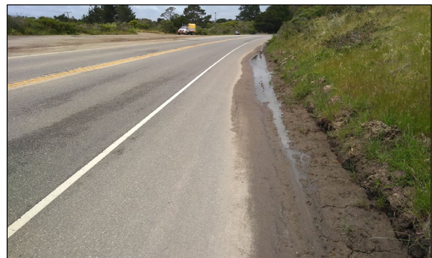
Figure 2.9: Example of drainage problem in cut (note moisture in wheelpaths).
