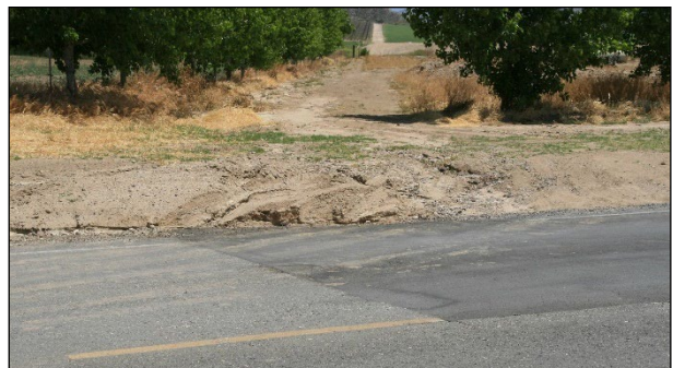
Figure 3.31: Access road drainage problems (note patch).
