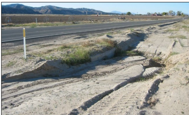
Figure 2.8: Example of blocked side drains and culvert.
