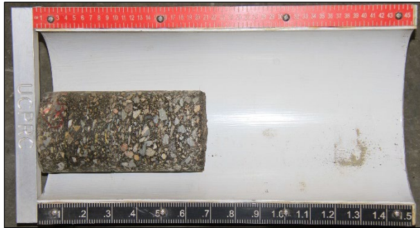
Figure 3.39: Core measurement of core with only asphalt concrete layers.
