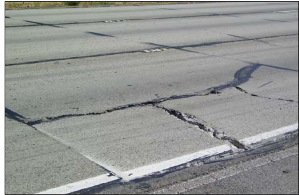
Figure 3.15: Jointed plain concrete slab with wide and spalled third-stage cracking (7).
