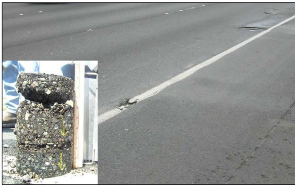
Figure 3.3: Cracking, pumping, & potholes from moisture damage in asphalt concrete layers. (a core from the section is shown on the inset photo)
