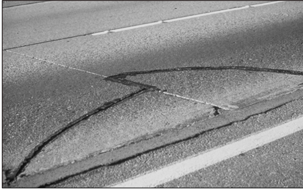
Figure 3.12: Corner cracks on jointed plain concrete pavement.
