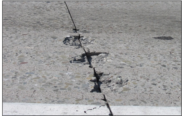
Figure 3.19: Spalled transverse joint between jointed plain concrete slabs.
