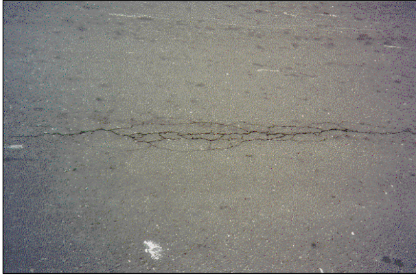
Figure 3.1: Initial fatigue cracking in wheelpath.
