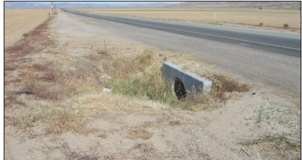
Figure 3.27: Blocked side drain and culvert.
