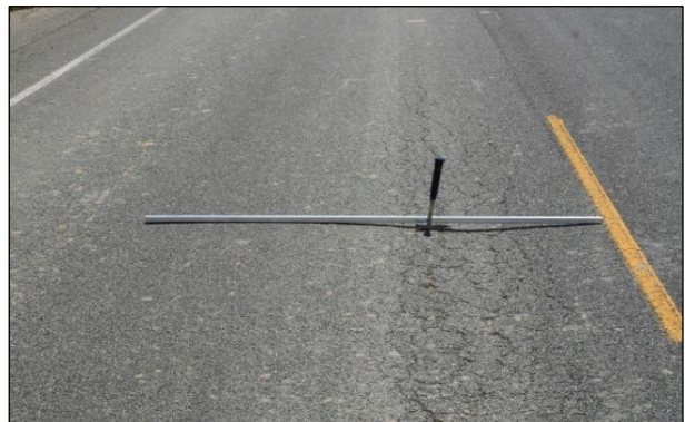
Figure 2.6: Example of rutting associated with base/subgrade failure.
