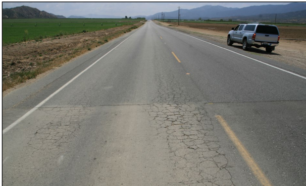
Figure 2.1: Example of early patch failure related to poor drainage.
