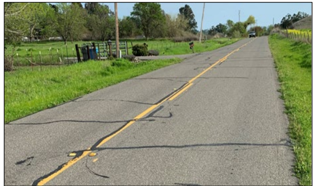
Figure 3.8: Sealed transverse oxidative-aging cracks (reflection confirmed with core).
