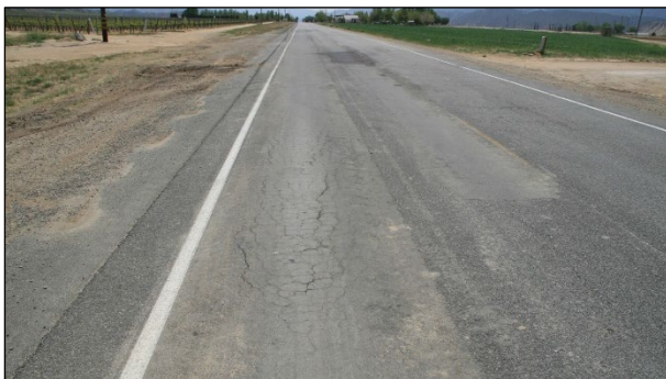
Figure 3.24: Early failure in wheelpath digout repairs.
