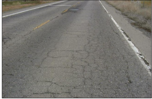
Figure 3.2: Severe fatigue cracking.
