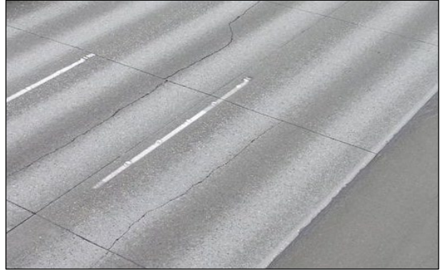
Figure 3.17: Longitudinal cracks on jointed plain concrete slabs.
