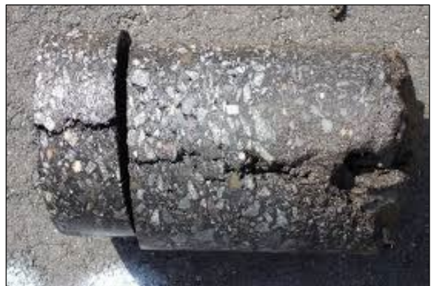
Figure 3.45: Debonded asphalt concrete with full-depth reflective crack.
