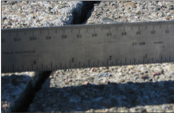
Figure 3.18: Faulting on jointed plain concrete slabs.
