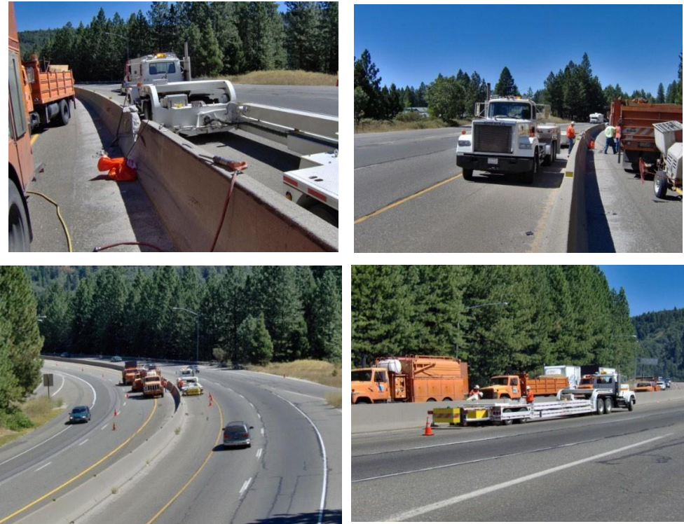
Figure 4.3: Median repair on a curved section of a highway (Courtesy of District 5).
