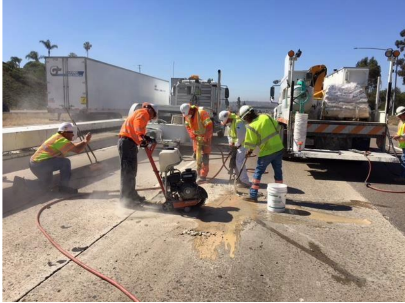
Figure 4.1: Balsi Beam provides cover for operating on the second lane (courtesy of District 11).
