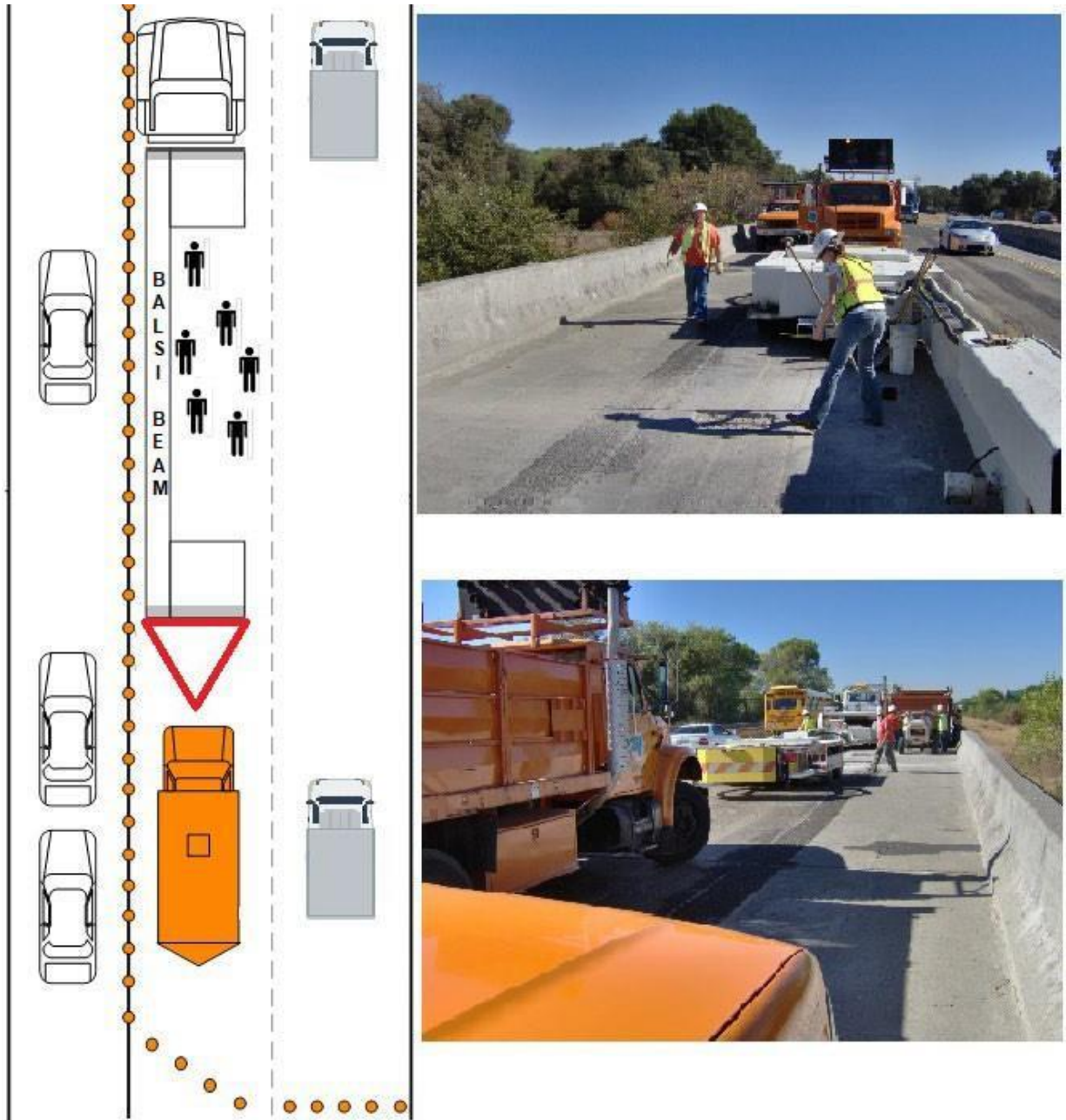
Figure A.3: Balsi Beam used in the second lane of the road. When used in the second lane, the first lane must be protected with an additional barricade truck. The first lane and second lane can be used to set up trucks carrying equipment/material. (Balsi Beam Kearny Mesa Bridge Maintenance Crew)
