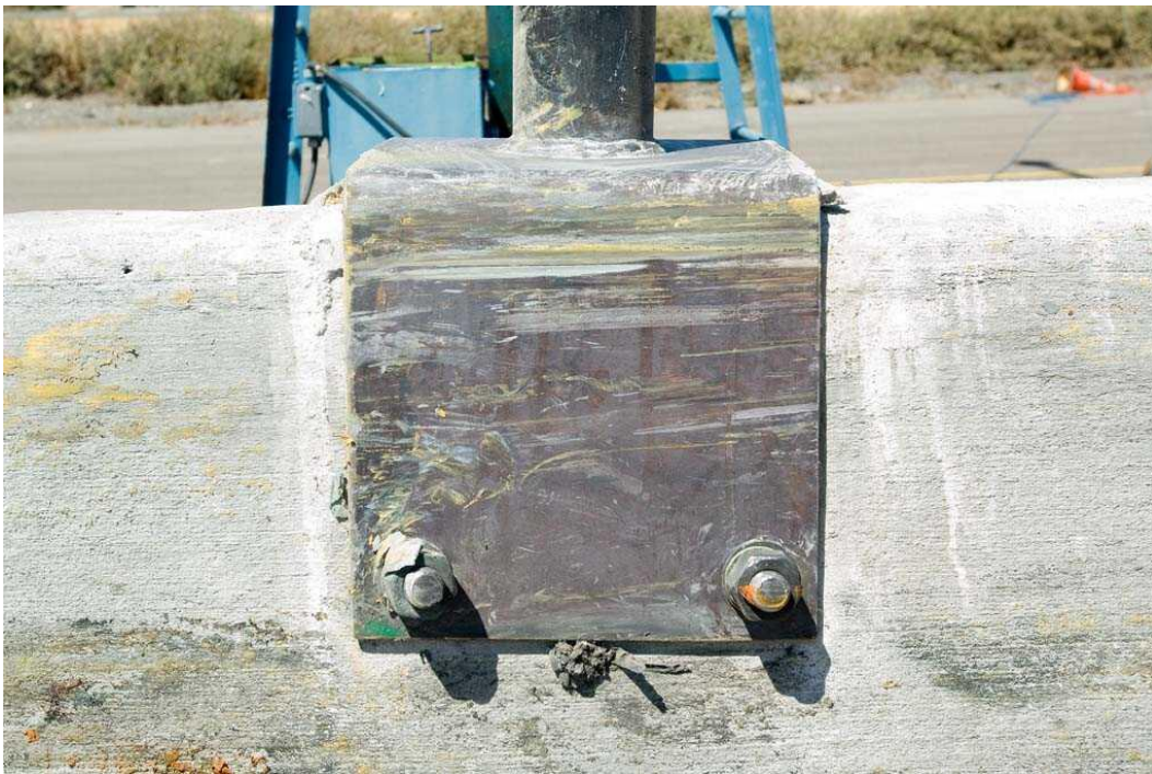
Figure 2-17 Signpost Saddle After Test
