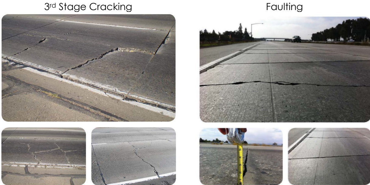
FIGURE 4. EXAMPLES OF DISTRESS FOR CONCRETE PAVEMENT
