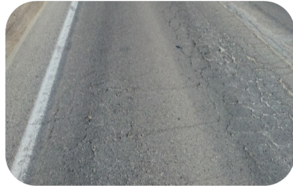
Alligator B Cracking
