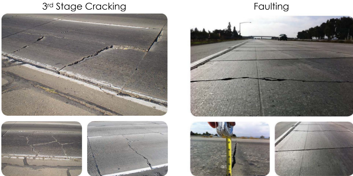
FIGURE 4. EXAMPLES OF DISTRESS FOR CONCRETE PAVEMENT
