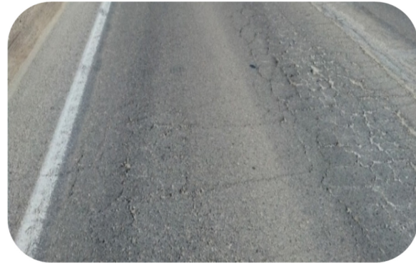
Alligator B Cracking
