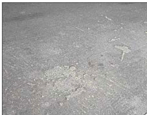
b) Delamination from a False Slurry
