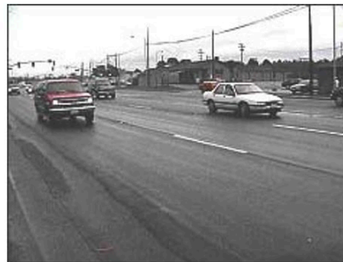
b) Poor-Quality Edges and Shoulder
