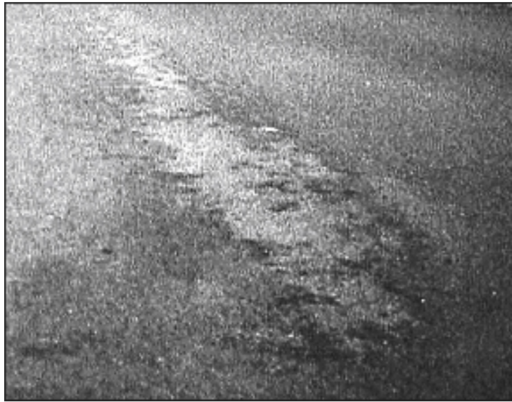
Figure 9-23 Traffic Damage Caused by Early Trafficking
