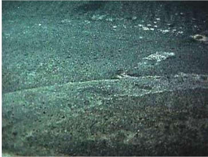
Figure 9-24 Damage Due to Post Application Heavy Rain with Shear
