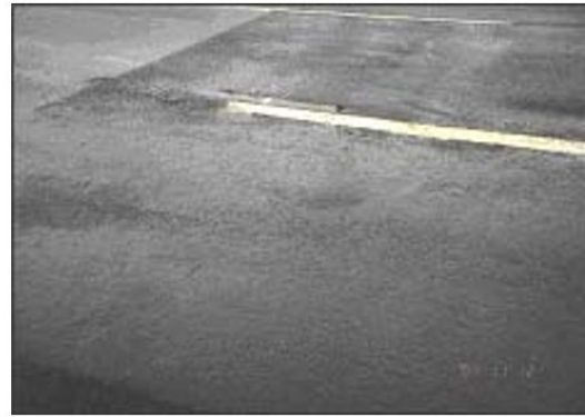
b) Poor-Quality Transverse Joint
