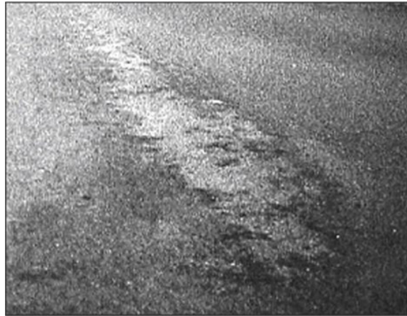
Figure 8-24 Traffic Damage Caused by Early Trafficking
