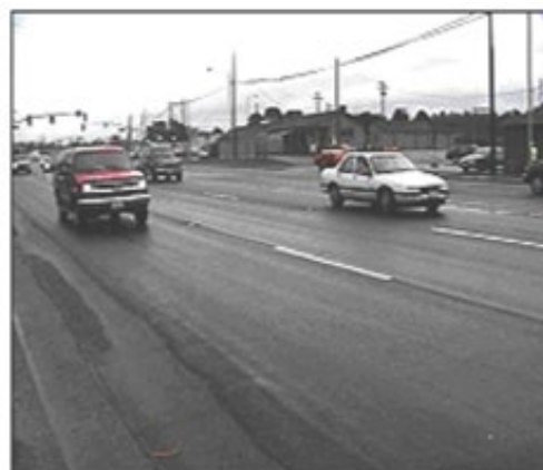
b) Poor-Quality Edges and Shoulder
