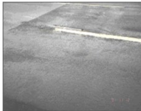
b) Low-Quality Transverse Joint
