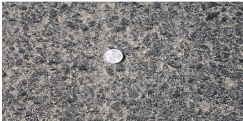
Figure 6-2 Suitable Surface, Heavily Aged Dense Graded HMA with Loss of Fines
