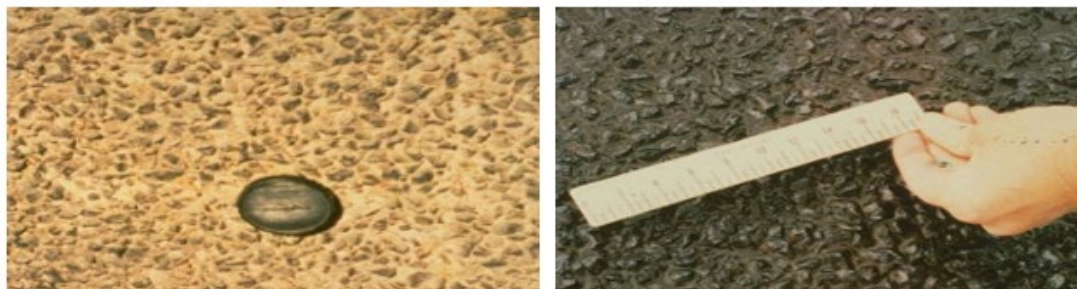
Figure 6-5 Chip Seal Before (Lt.) and After Fog Seal or Flush Coat (Rt.)
