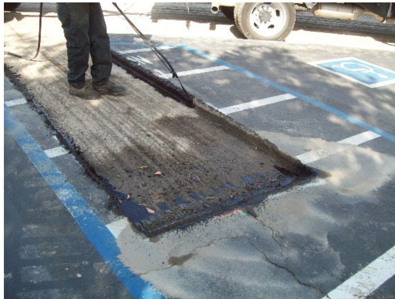
Figure 5-14 Existing HMA Removed at the Cut Lines of the Patch, and Tack Coat Applied on Vertical Faces of the Cuts
