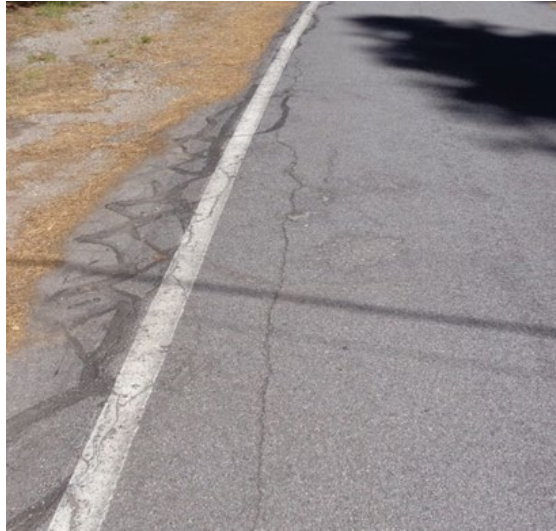
Figure 5-18 Example of Edge Cracking of a Pavement
