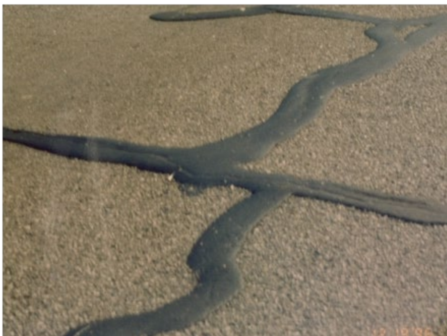
Figure 4-23 Excessive, Raised, Bumpy Overband
