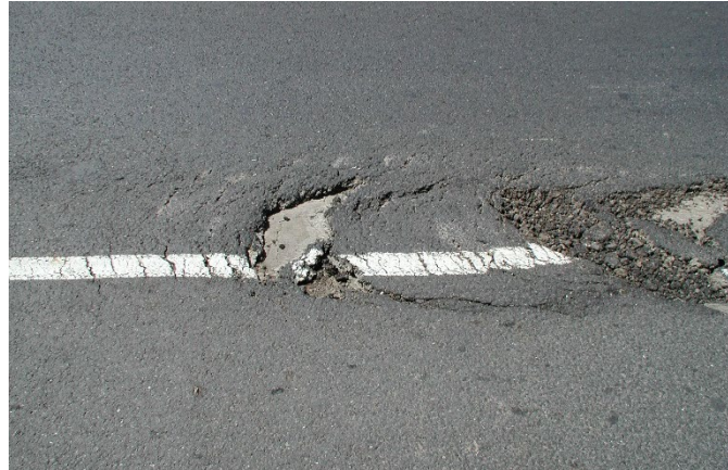
Figure 4-8 Advanced Slippage Cracking
