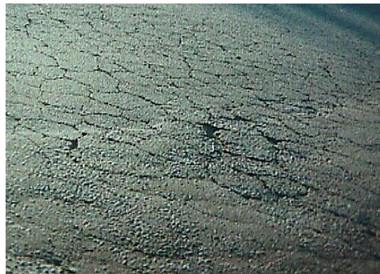
Figure 4-2 Alligator (Fatigue) Cracking
