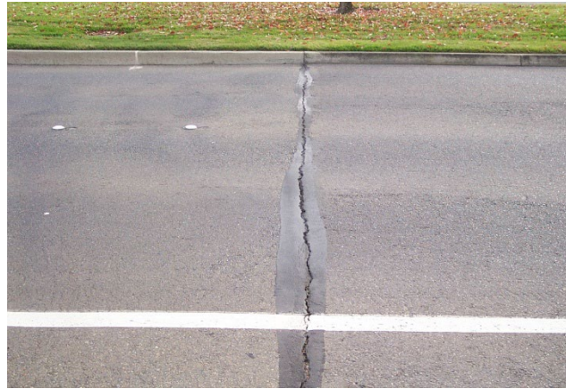
Figure 4-6 Transverse Reflection Cracking
