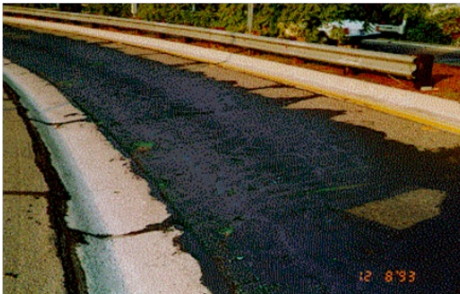
Figure 4-22 Excessive Multiple Treatments
