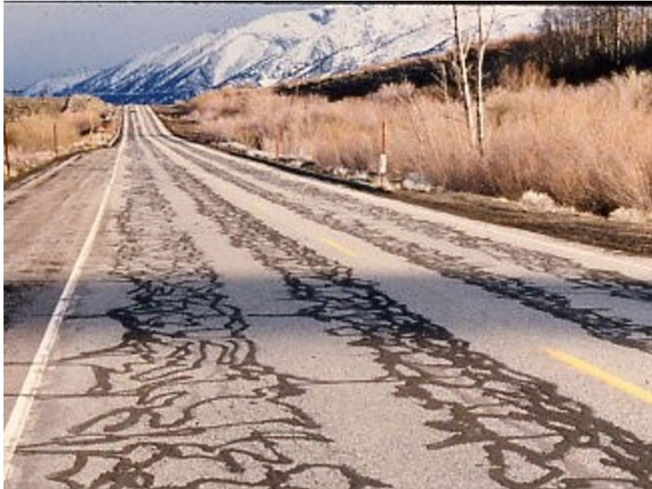
Figure 4-24 Sealing of Alligator Cracking (Not Recommended)
