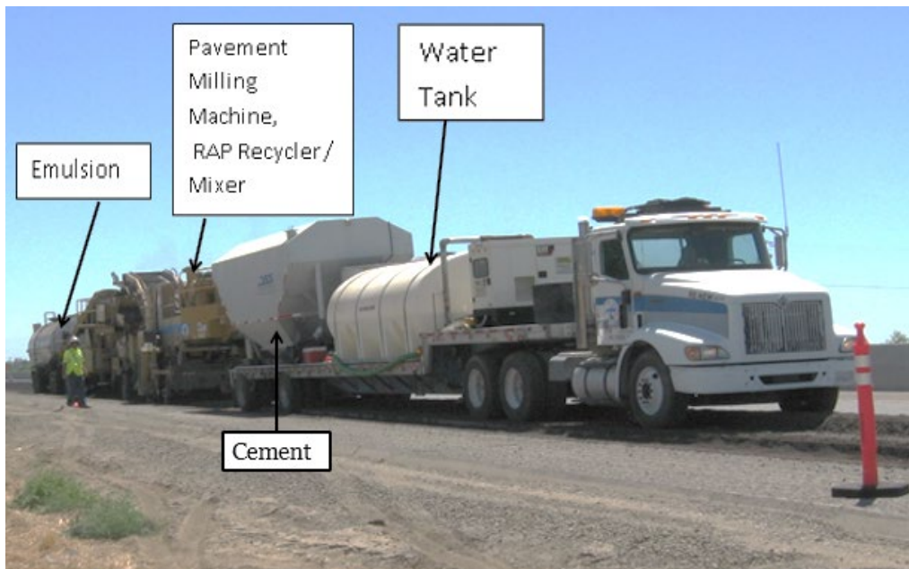
Figure 14-3 PDR Equipment Train (Courtesy CP2 Center)
