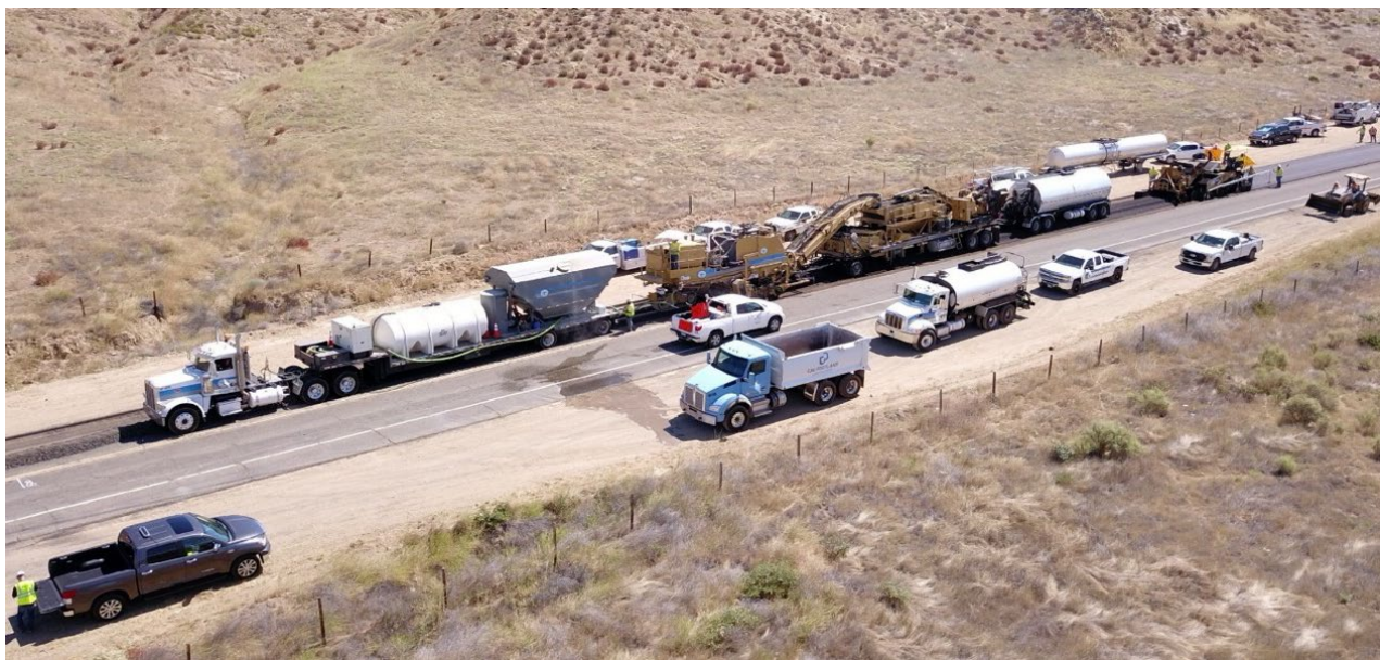
Figure 14-5 PDR Full Equipment Train with Paver (Courtesy Mike Concannon, Pavement Recycling Systems, Inc.)
