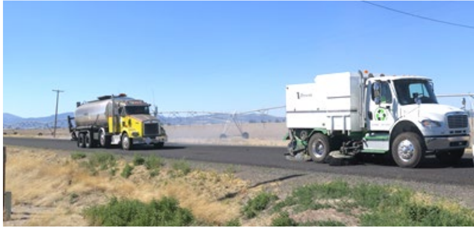
Figure 10-15 Self-Contained Sweeper Truck on Right
