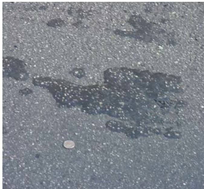
Figure 1-28 Bleeding/Fat Spot (Seal Coats)
