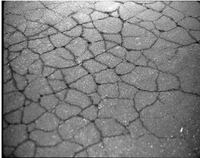
Localized High Severity Alligator Cracking
