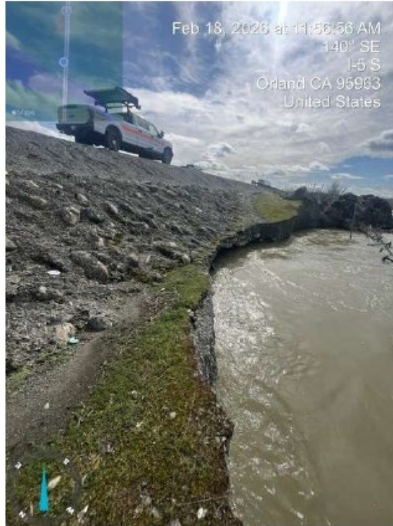
GLE-5-PM 27.05: Damaged fence embedded into creek and loss of embankment material
