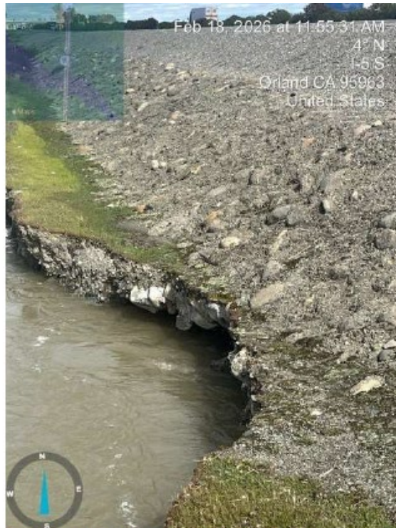
GLE-5-PM 27.05: Loss of embankment material caused by recent storm
