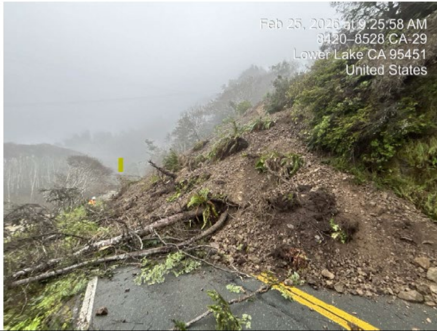
MEN-1-31.15: Landslide debris blocking both lanes of travel, resulting in full highway closure
