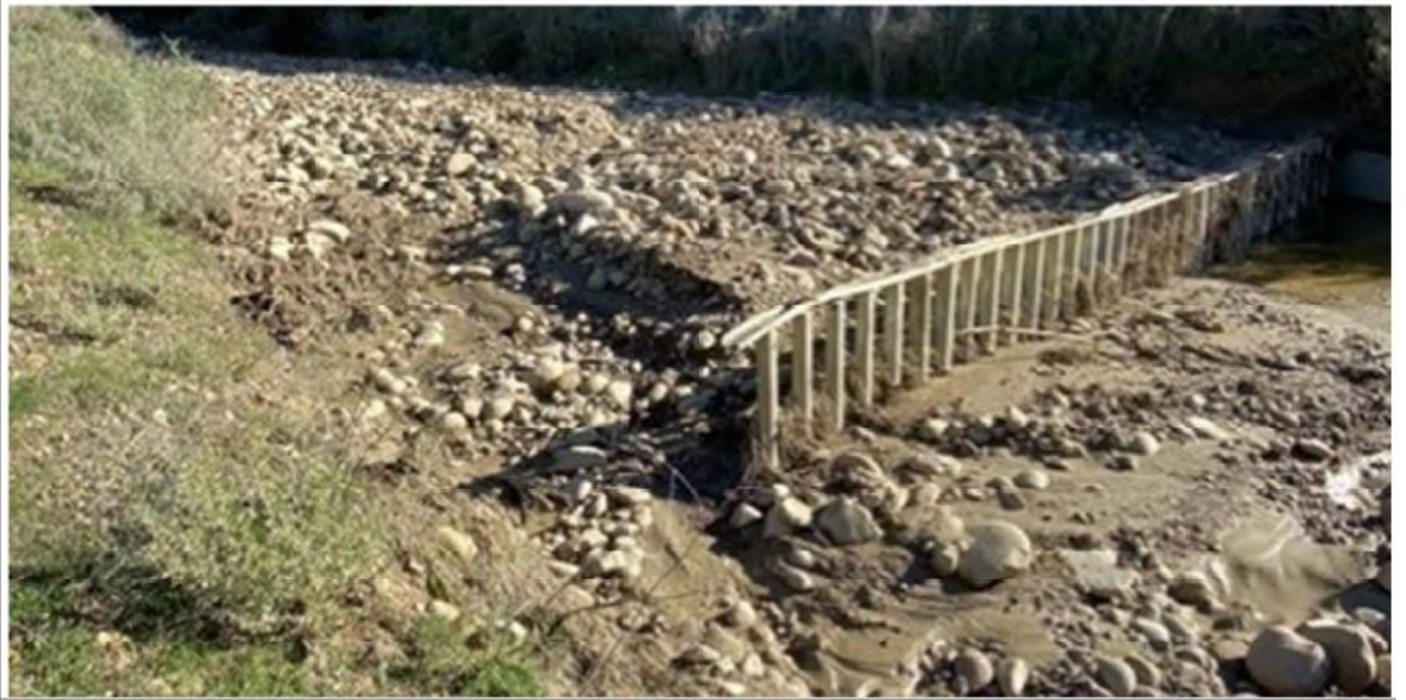
This Photograph Shows: Debris flow from the canyons filled the detention basin. The material has stopped at the debris rack but is at near capacity (VEN 101 at PM 32.67) Picture #3
