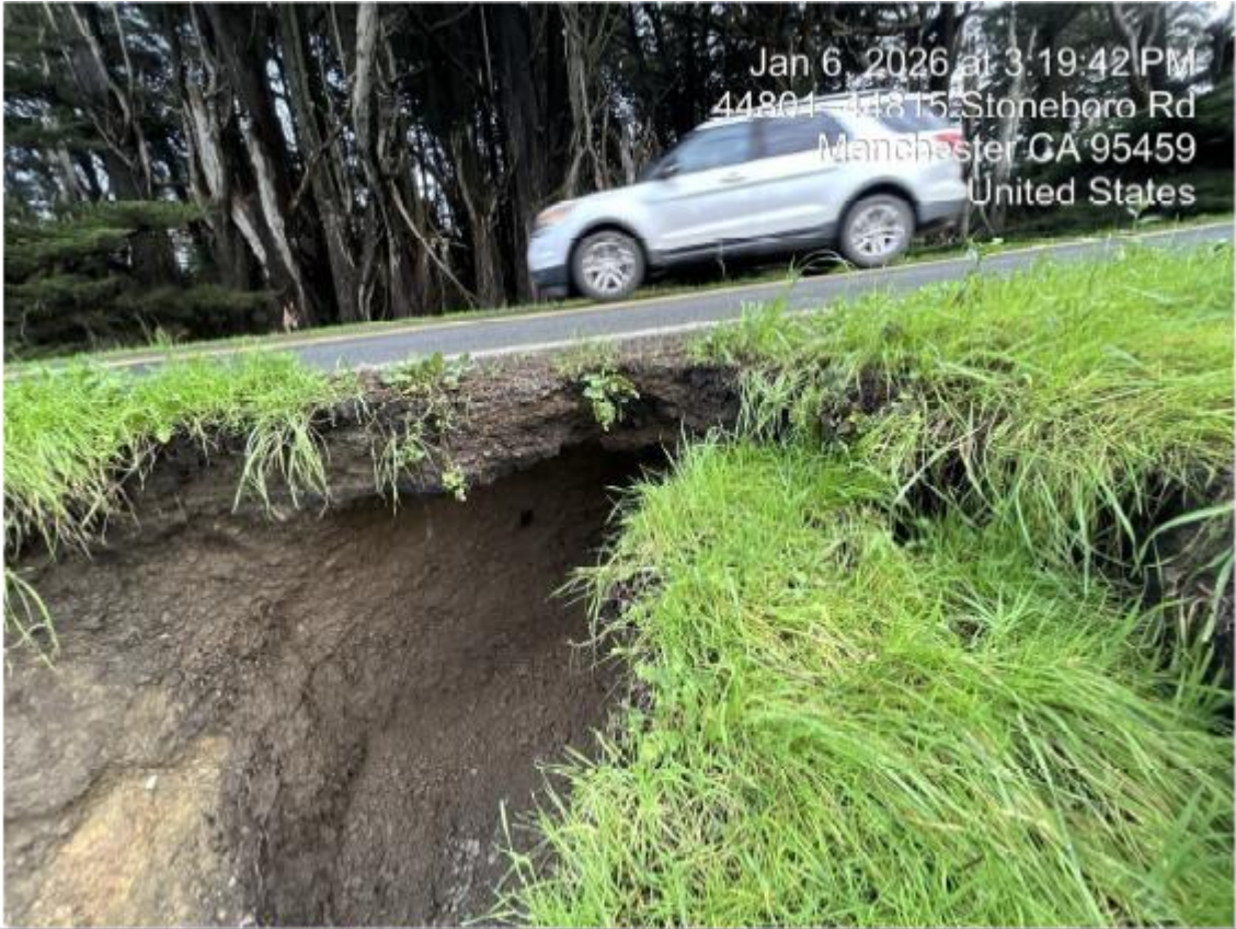
Roadway damage caused by failed drainage system (MEN-1-19.64)
