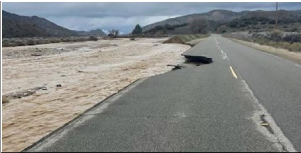
This Photograph Shows: Creek eroded berm and side slope resulting in a partial collapse of the roadway on VEN 33 at PM 50.0
