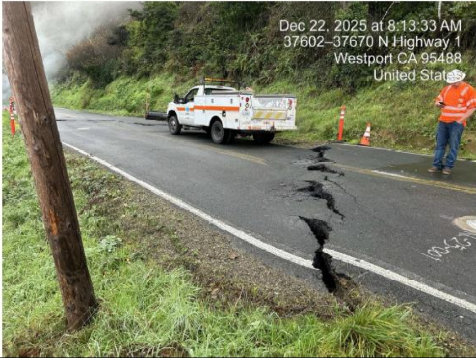
: Pavement cracking across both lanes caused by landslide and roadway slipout (MEN-1-78.2)
