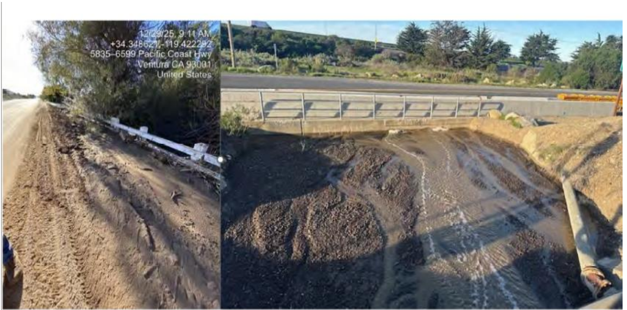
This Photograph Shows: VEN-1-PM 28.2 - Clogged drainage system and roadway edge with mud and debris. Picture #3
