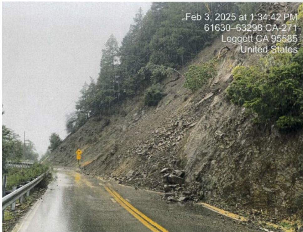
This Photograph Shows: MEN-271-2.4-2.5 PM Landslide
