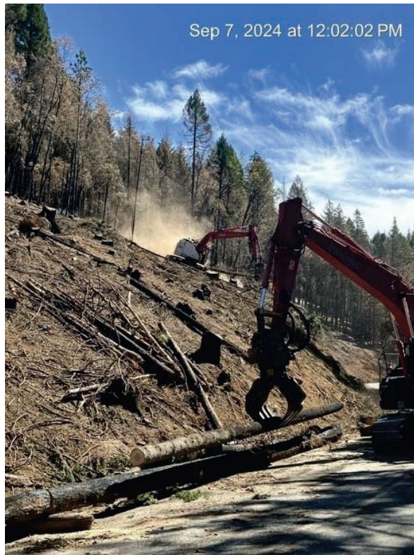
03-BUT-32 – Park Fire -typical Damages Park Fires Butte/Tehama Counties
