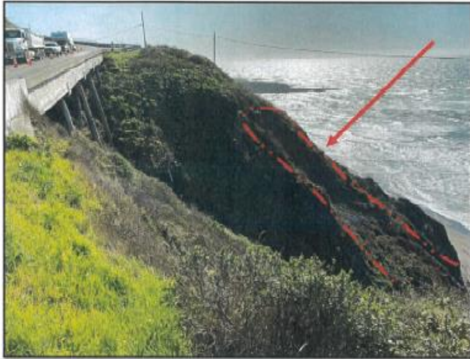
This Photograph Shows: MEN 1 PM 75.0 - Landslide adjacent to Blue Slide Gulch Viaduct (10 - 0166) as a result of rainfall and high surf.
