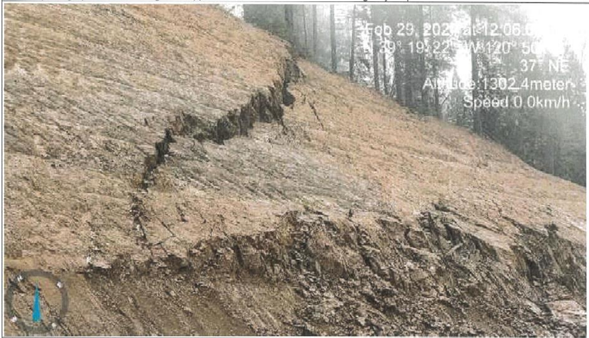
This Photograph Shows: NEV-20-30.1 Slide material from slope and large diagonal crack caused by slip out/undermining of the slope.
