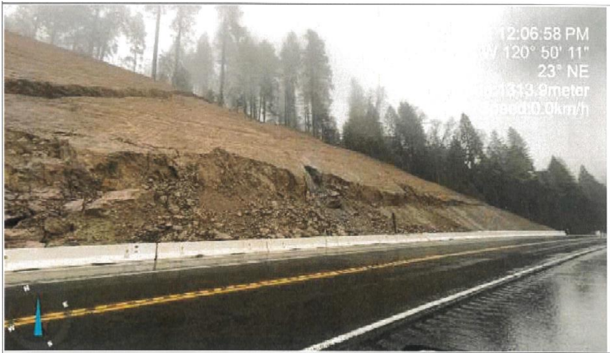
This Photograph Shows: NEV-20-30.1 Side view of slide material and large diagonal crack/undermining of the slope.
