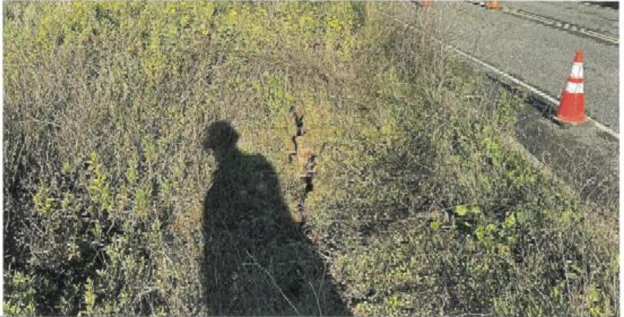
This Photograph Shows: Multiple surface cracks on the side slope
