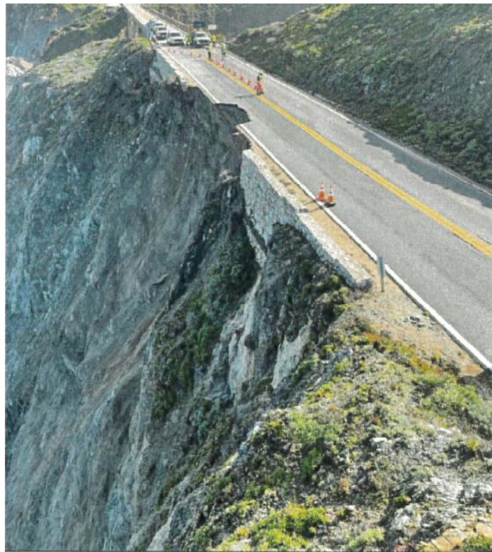
05-MON-1 Typical Masonry wall failure, PM 60.0
