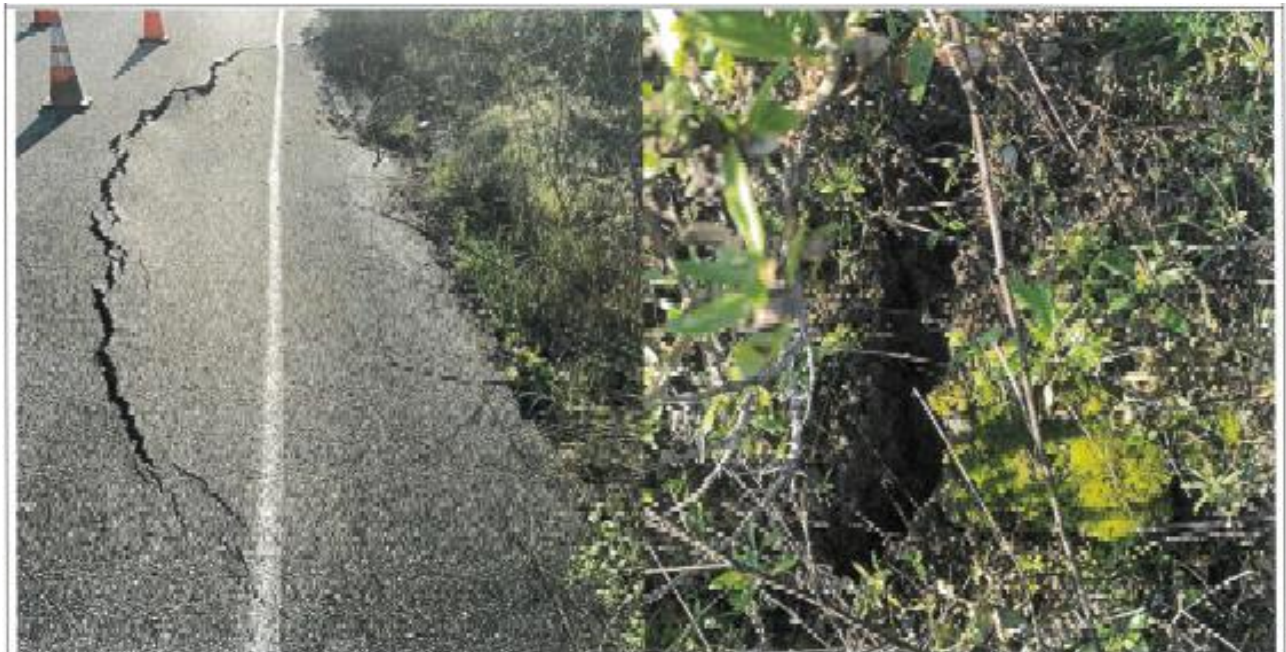
This Photograph Shows: (Left) The slope failure has caused the right side of the curb/shoulder lane to crack and slide down the slope. (Right) large cracks and separation at the surface of the side slope that is sliding down.
