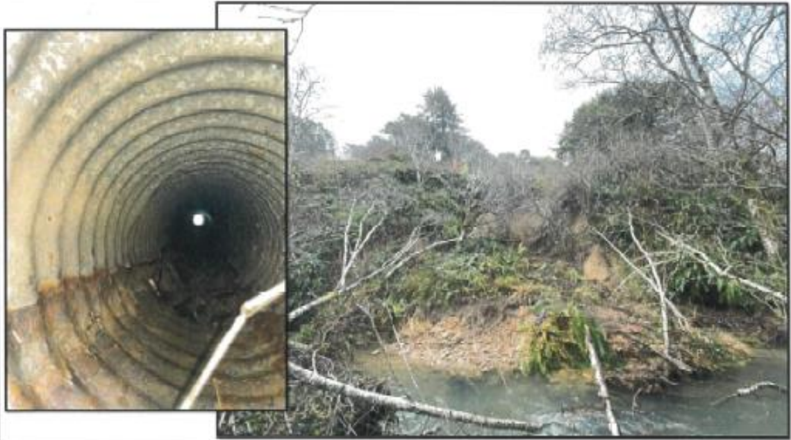
This Photograph Shows: MEN 1 PM 78.25 - Large slipout resulting in roadway settlement and culvert damage. A geotech investigation is needed for this location.
