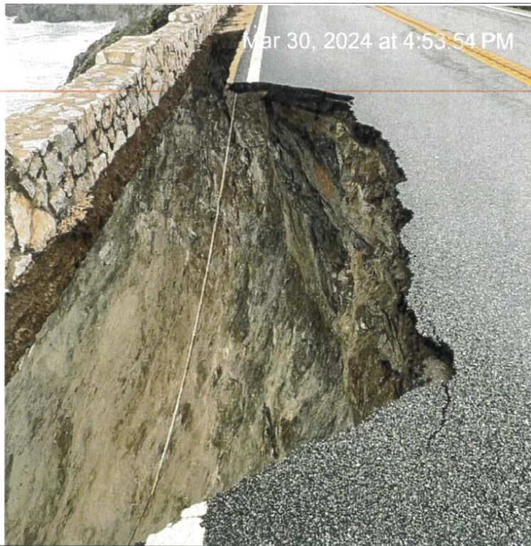
05-MON-1 Typical roadway/pavement damage, PM 60.0
