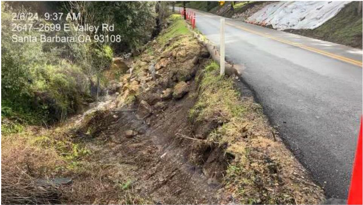
This Photograph Shows: Location 6: 05-SB-192-11.65 Slipout and erosion threatening the roadway.
