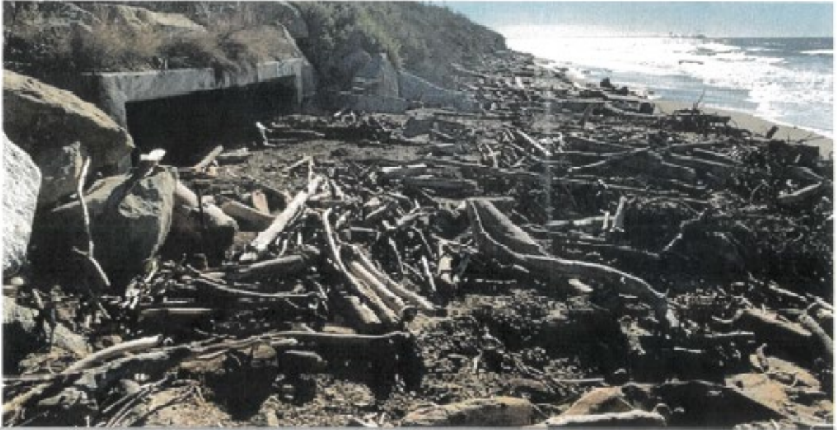
This Photograph Shows: Typical exit of a concrete box culvert blocked with mud, sediment and driftwood (at System Number 521010004187 at ET 1).
