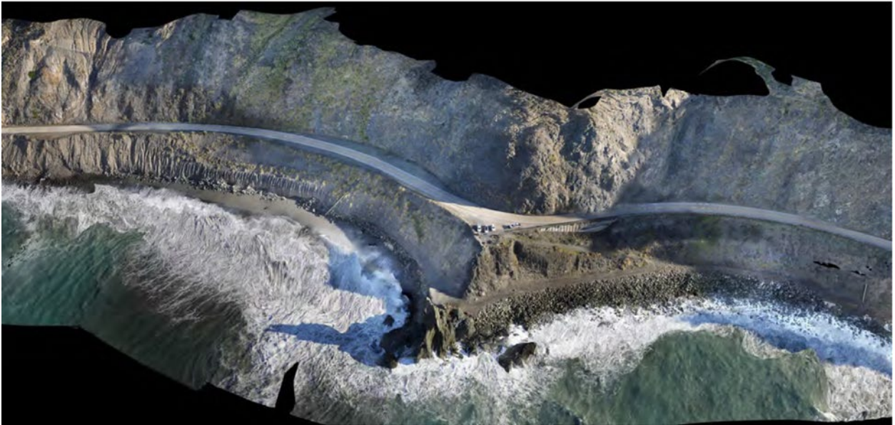
This Photograph Shows: MON-1-7.1/7.9 Drone image showing RSP loss
