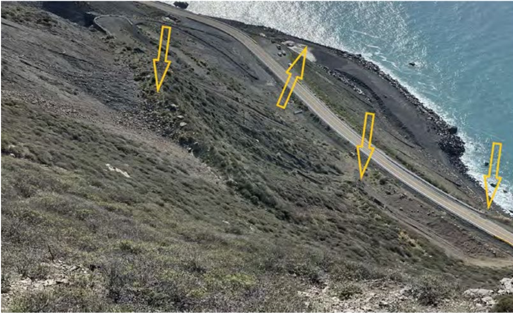
This Photograph Shows: MON-1-8.7/9.2: Mud Creek: Degraded catchment access road, filled catchment, rockfall damaged pavement and RSP loss
