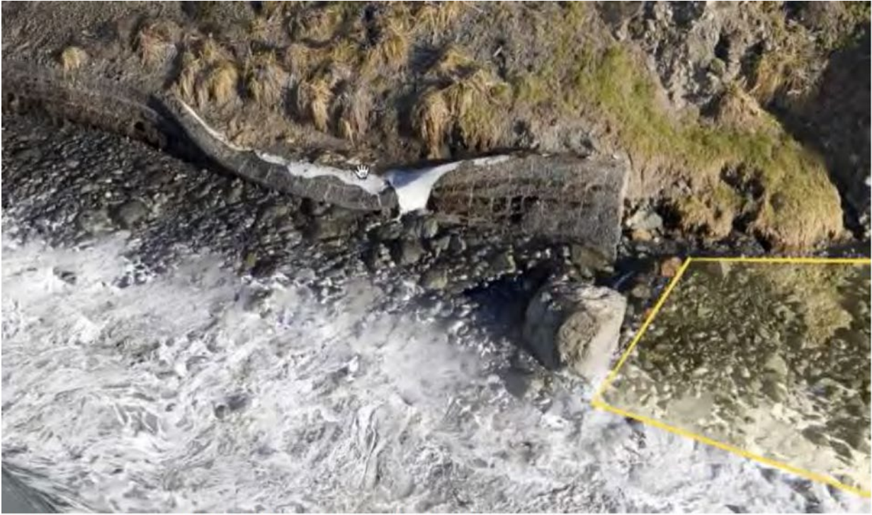
This Photograph Shows: MON-1-7.1/7.9 Collapsed gabion baskets
