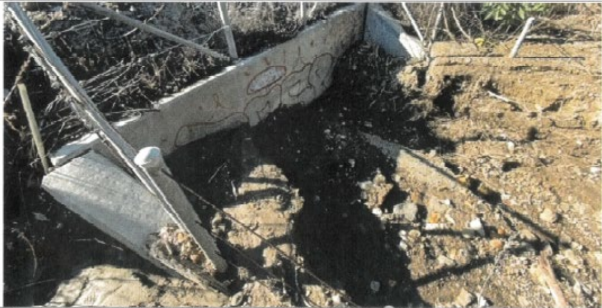
This Photograph Shows: Typical blocked entrance of a concrete box culvert filled with mud and sediment from the mountain side. The debris flow was stopped due to the exit and inside of the box culvert being filled with debris (at System Number 521010004187 at ET 3).
