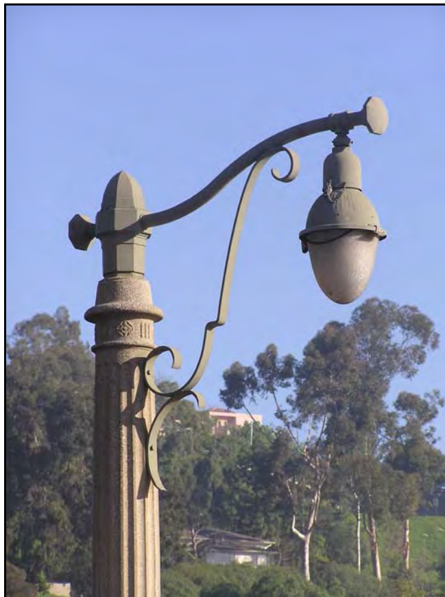
Photograph 4: Light detail, facing northeast, March 2004
