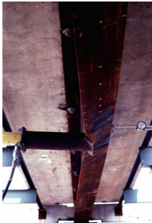
Figure 7-31. Category T-Damage (FHWA, 2008)
