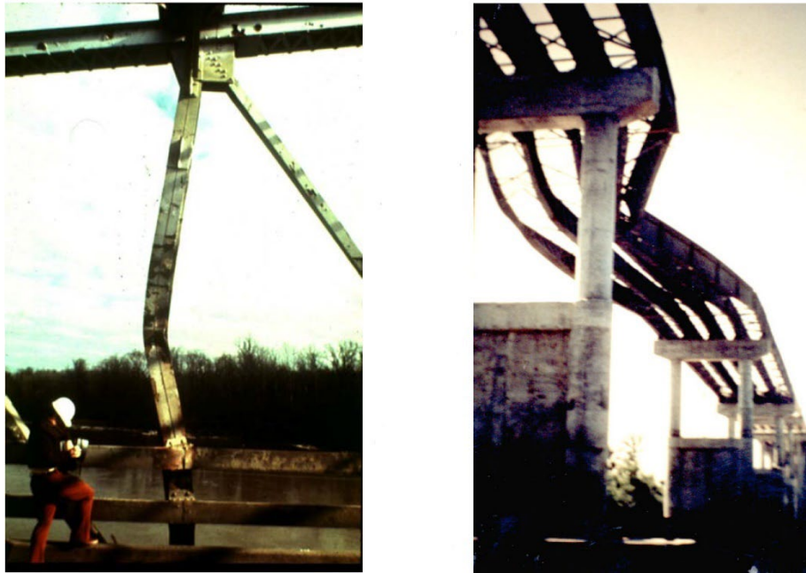
Figure 7-30. Category W-Damage (FHWA, 2008)
