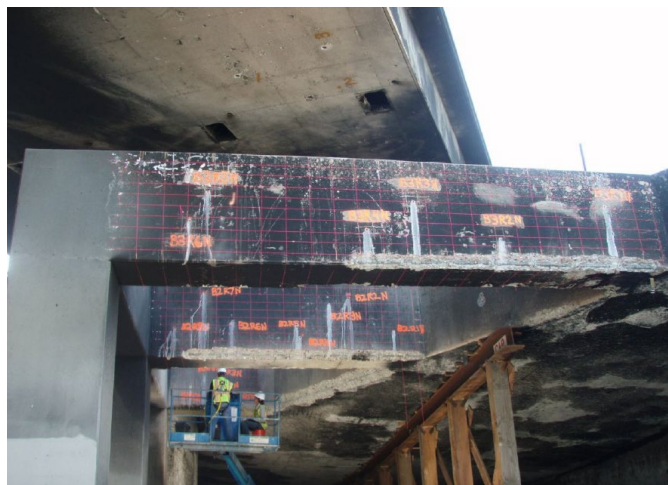
Figure 7-24. Fire Damage to SR-2/I-5 Connector Tunnel
