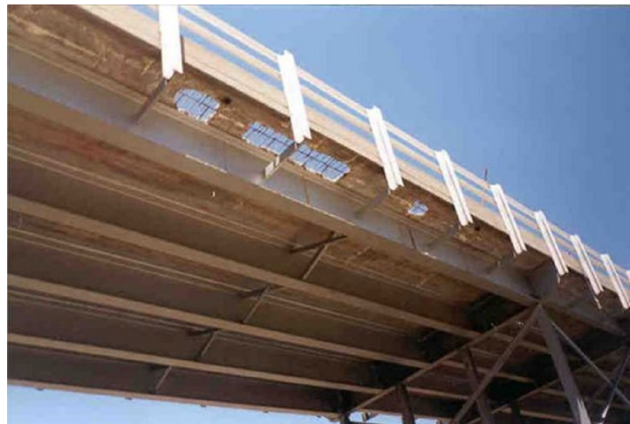
Figure 5-1. Example of Bridge Deck Damage
