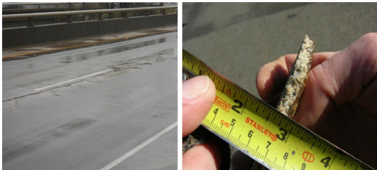
Figure 5-55. Thin Layer of Polyester Concrete Overlay that Failed
