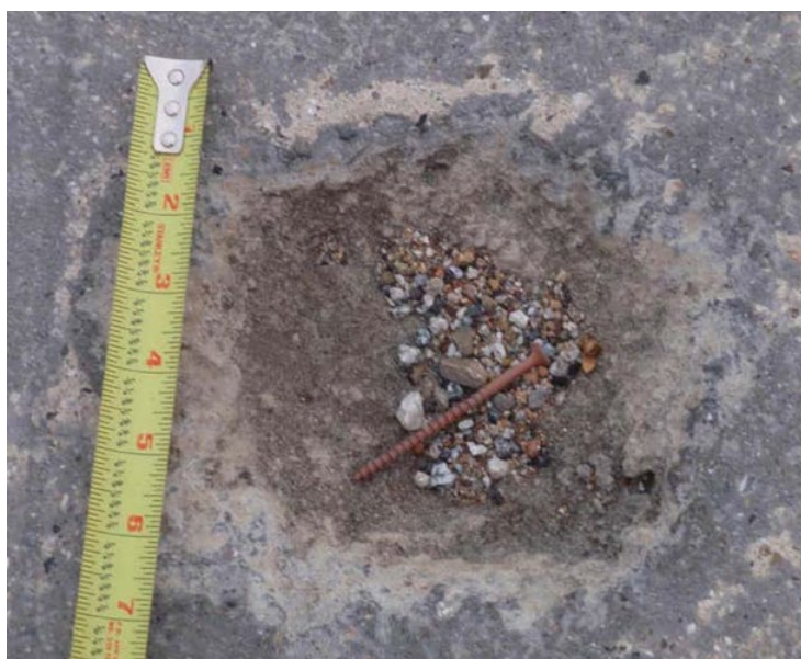
Figure 5-4. Severe Bridge Deck Scaling (Small Pothole)
