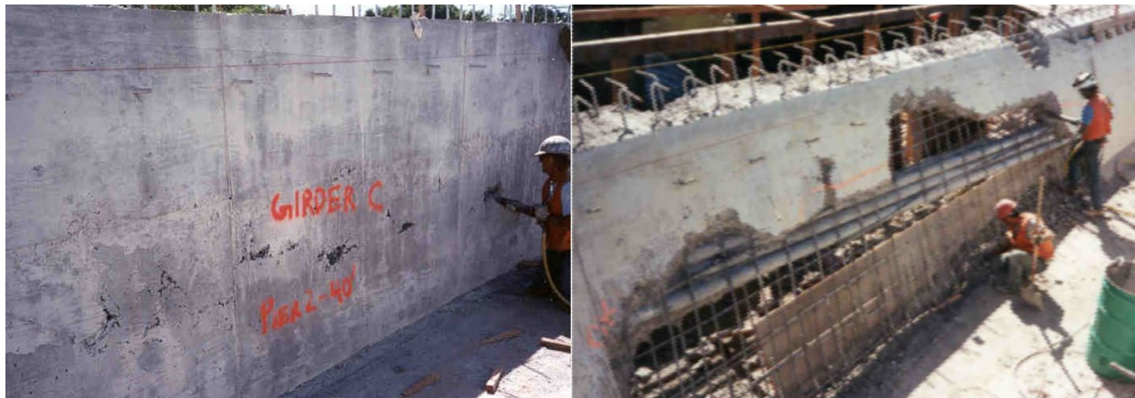
Figure 5-2. Rock Pocket Damage- both Minor and Major
