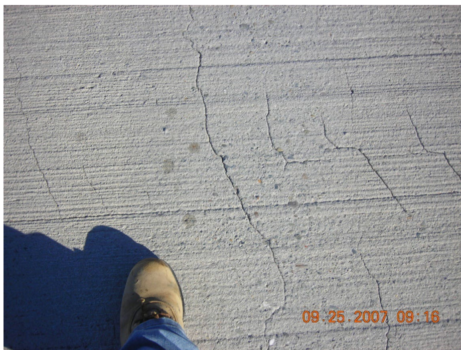
Figure 5-40. Bridge Deck Cracks
