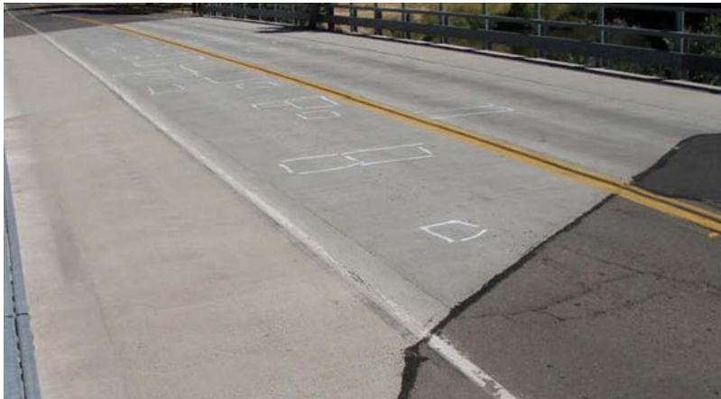
Figure 5-16. Locations of Unsound Concrete Identified by Chaining Marked on Bridge Deck
