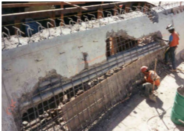
Figure 5-32. Large Voids in Bridge Girder
