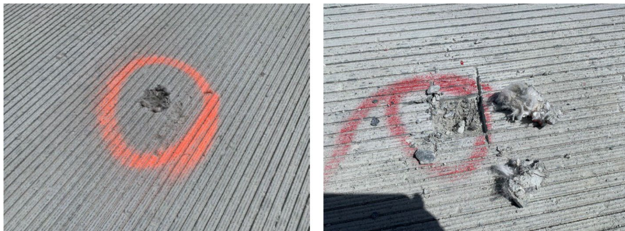
Figure 5-35. Required Patching in New Bridge Deck
