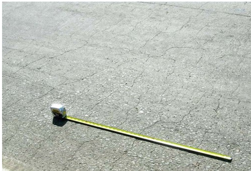
Figure 5-3. Map Cracking of a Bridge Deck
