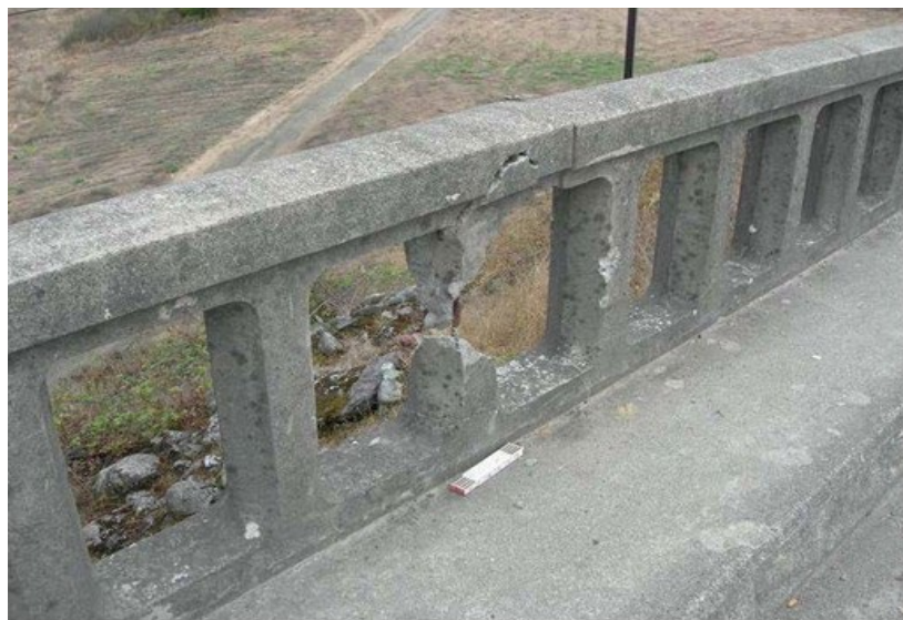
Figure 5-6. Surface Spalling Caused by Vehicle Impact
