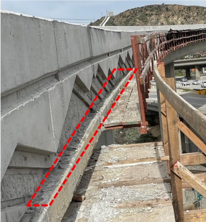
Figure 4-34. Support at Edge of Bridge Deck that Was Utilized During Barrier Forming
