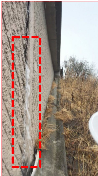
Figure 4-20. Water Pouring out of Joint Due to Defective Water Stop
