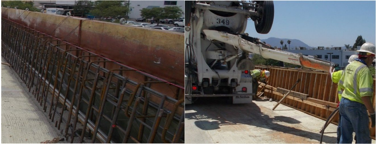
Figure 4-32. CIP-FF Forming: No PC Mortar Block Is Attached to Traffic Side Rebar
