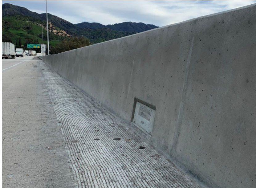
Figure 4-9. Bridge Barrier Pull Box
