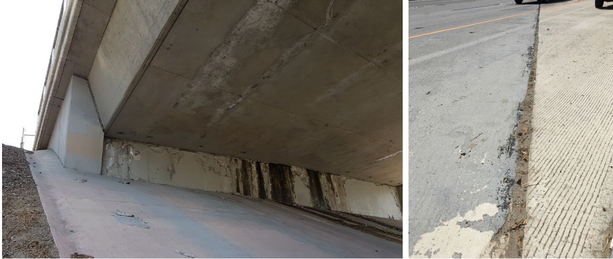
Figure 2-2. Consequence of Joint Seal Failing
